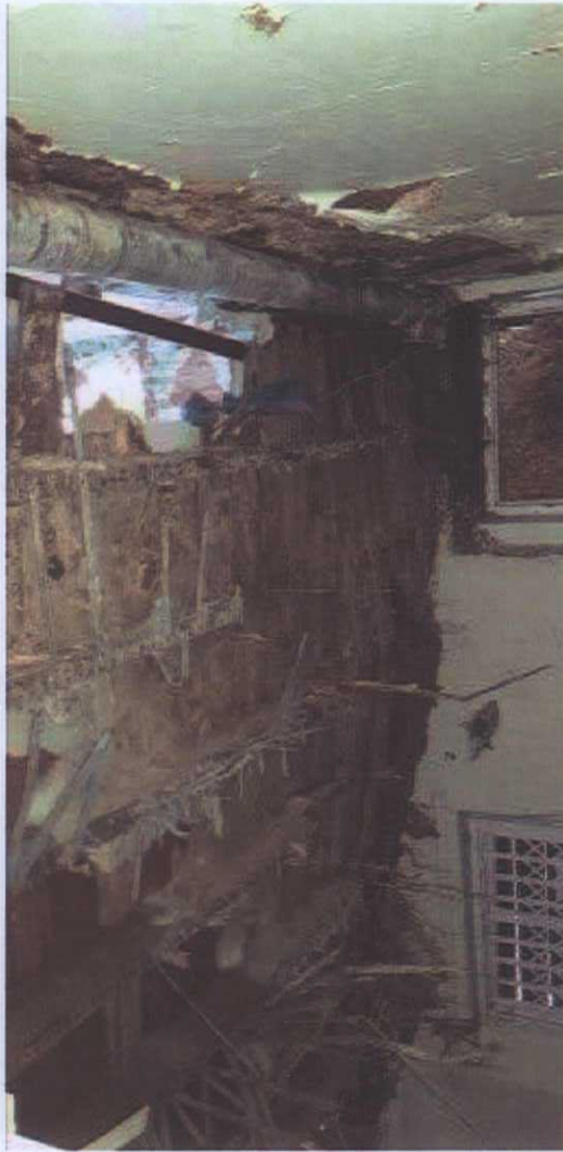
Collapsed ceiling & floor above
