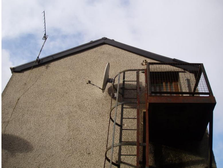
Eastern facing gable, gaps beneath UPVC fascia
