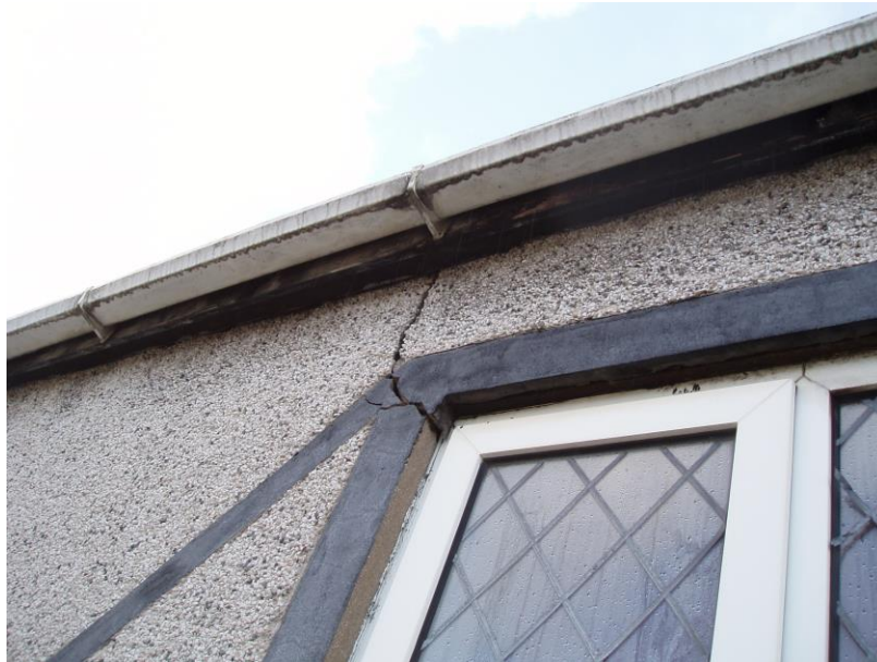
The large crack above the window
