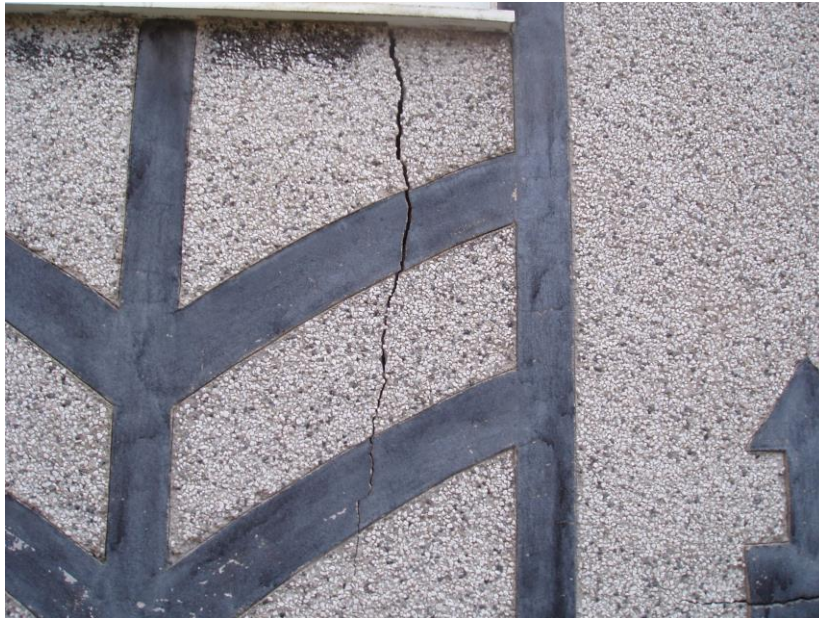
The large crack below the window on the second floor facing the main road
