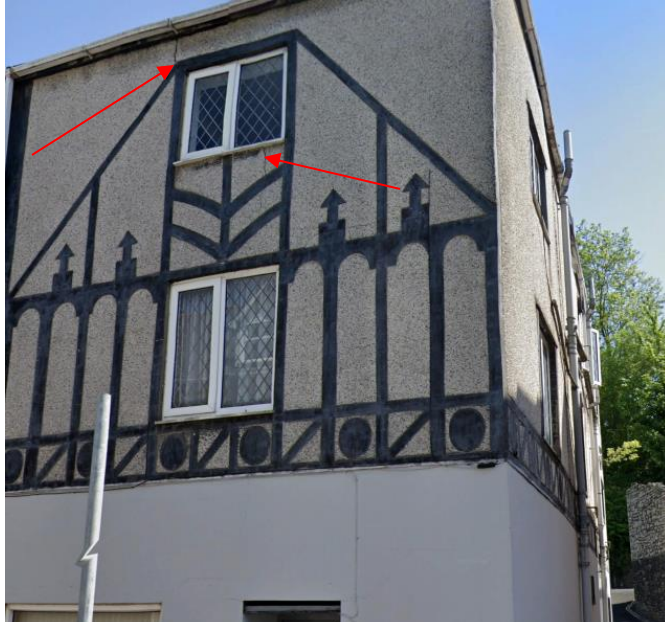
Front elevation showing large cracks in render (photo Google Earth).
