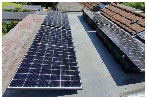
2 IMAGE OF SOLAR PV PANELS
