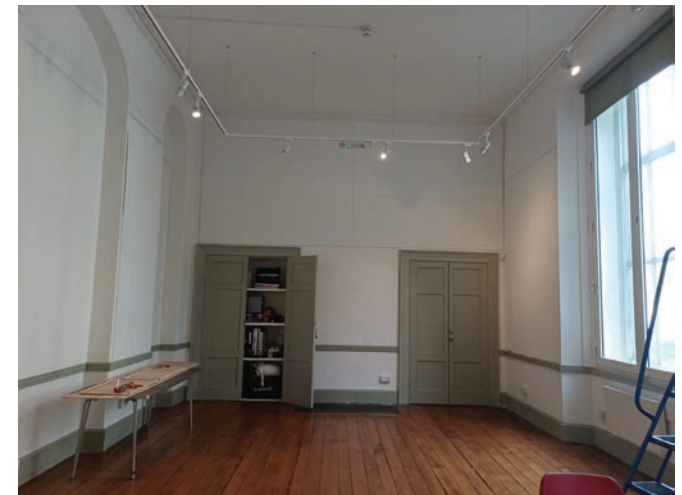
0.54 - Play room Track to be replaced like-for-like
