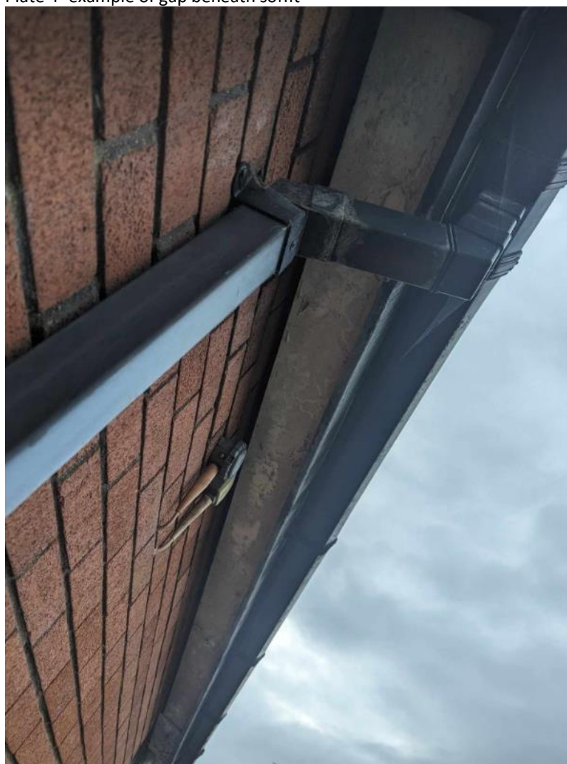
Plate 4- example of gap beneath soffit
