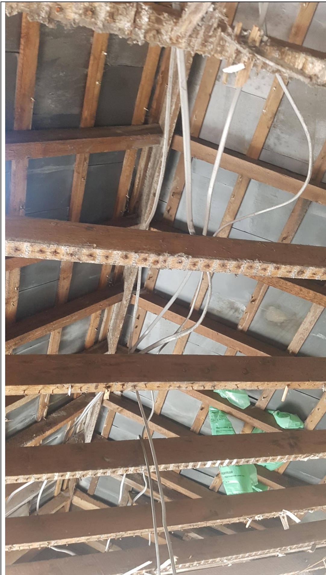
Photo 5. Underside of the roof covering, offering very small and poor roosting space over rafters.
