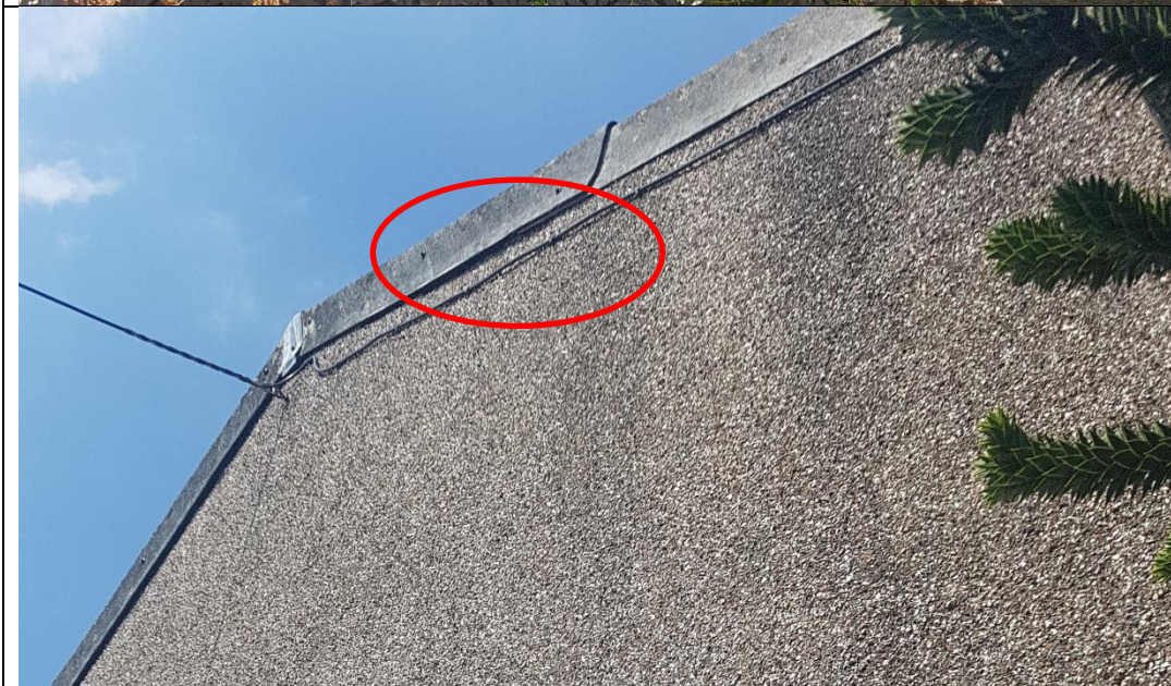
Photo 4. Side gable end (east) with small gaps at the barge board. Likely bat emergence point highlighted.
