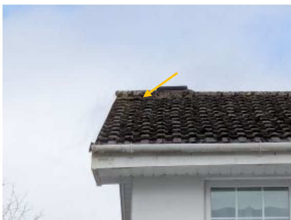
Building A – Southern elevation – PFF – Raised tiles
