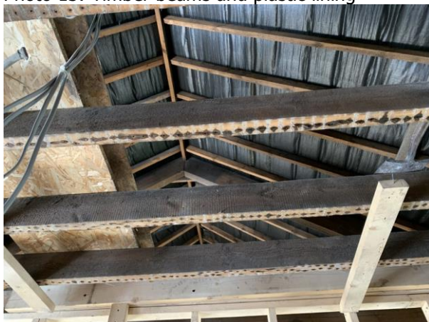
Photo 13: Timber beams and plastic lining
