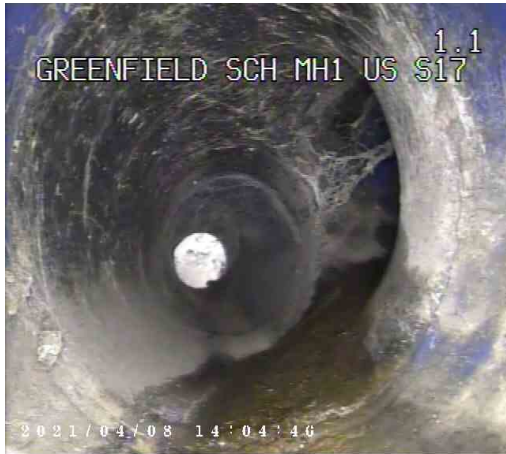
S17X_089b7654-ac54-43b0-a985-7d4709dd27fd_20210409_111310_415.jpg, 00:00:27, 1.20 m Junction at 3 o'clock, diameter: 150mm
