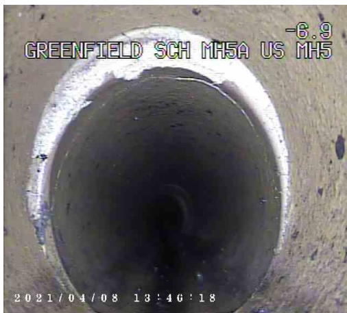
MH5X_66ca5f3c-a5ba-4cae-84ed-91cc88a78fdc_20210409_120404_401.jpg, 00:00:49, 7.00 m Joint displaced, medium
