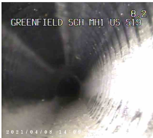
S19X_19c7ea18-c9f5-4cb1-8efc-64b29e25f29c_20210409_113031_413.jpg, 00:00:37, 8.00 m Settled deposits, coarse, 10% cross-sectional area loss, start
