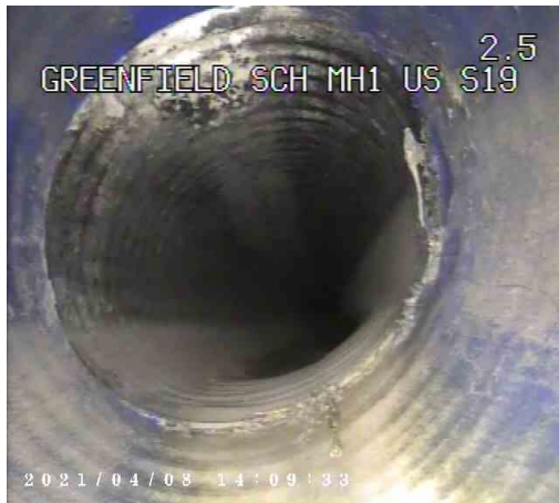
S19X_2070d7b8-d2cf-4c01-9172-b5b239d22960_20210409_112421_670.jpg, 00:00:12, 2.70 m Shape changes to oval, new size(s), 130mm high, 180mm wide, Pipe been squashed at bottom on the joint
