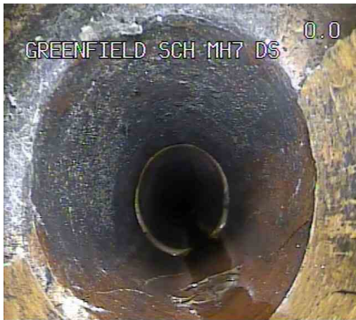
MH7X_b3d17391-9ac9-4437-ad4c-0bd7297b8cd9_20210409_131057_843.jpg, 00:00:00, 0.00 m Cracks, multiple from 3 o'clock to 9 o'clock
