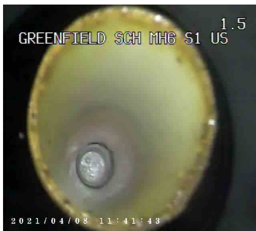
S1X_d1463d36-f64a-4ed6-8c1a-95be66f60feb_20210409_13 0303_076.jpg, 00:00:13, 1.50 m Survey abandoned, End of line in building.
