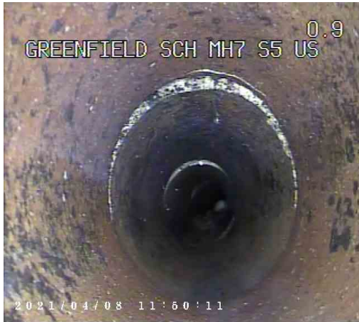
S5X_1c40c8f5-375d-4011-b65b-048b5e0933bf_20210409_13 2324_234.jpg, 00:00:07, 0.90 m Crack, circumferential at joint from 11 o'clock to 2 o'clock
