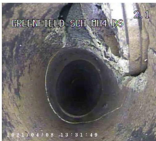
MH4X_888a0a1b-f5d6-4178-8084-9966d7f5f239_20210409_15543_842.jpg, 00:00:27, 2.20 m Hole in drain or sewer at joint at 12 o'clock, Hole above connecting pipe.
