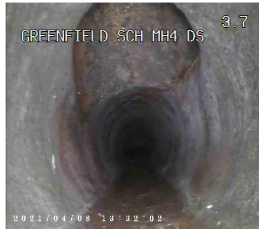
MH4X_2c47259a-7974-4135-a027-93da851b07c5_20210409_115705_772.jpg, 00:00:33, 3.80 m Junction at 12 o'clock, diameter: 100mm
