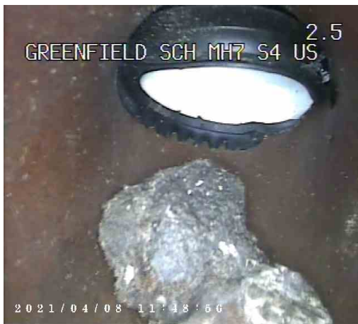
S4X_f9f919cd-5e90-4493-bac2-2d880f9852d1_20210409_13 2126_617.jpg, 00:00:41, 2.50 m Survey abandoned, End of line in building.
