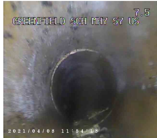
S7X_95626faf-779e-457a-8c7d-22ee80fa5031_20210409_133340_128.jpg, 00:00:30, 7.50 m Settled deposits, coarse, 5% cross-sectional area loss, start
