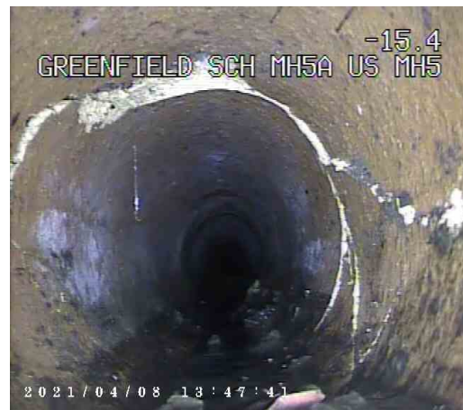
MH5X_325b1eac-ae86-49ed-895e-ded158ba6d0b_20210409_121752_672.jpg, 00:02:06, 15.10 m Crack, circumferential from 12 o'clock to 12 o'clock
