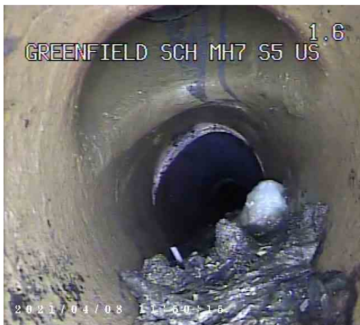
S5X_2742bc33-e987-4a5b-a546-aa8244d85aa1_20210409_1 32356_896.jpg, 00:00:11, 1.80 m Junction at 11 o'clock, diameter: 100mm
