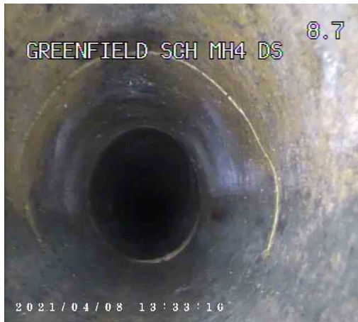
MH4X_739ae0a7-c8ac-4b7b-9a3c-6cac798f8d48_20210409_115924_634.jpg, 00:01:54, 8.90 m Crack, circumferential from 12 o'clock to 12 o'clock
