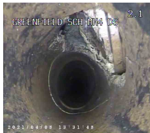
MH4X_cd588f8e-c44c-4a89-9936-6f002b1aa157_20210409_115614_618.jpg, 00:00:26, 2.30 m Crack, circumferential from 4 o'clock to 11 o'clock
