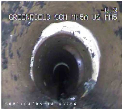
MH5X_ed2a13a7-1ff5-4519-9d26-d6a8b7d03c89_20210409_121031_657.jpg, 00:00:56, 8.00 m Joint displaced, medium
