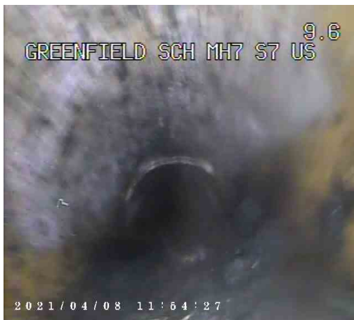
S7X_af4ce3c3-fa8c-4191-8308-354cad624a1d_20210409_133458_768.jpg, 00:00:39, 9.60 m Settled deposits, coarse, 5% cross-sectional area loss, start
