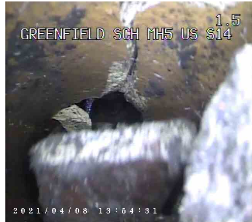
S14X_8eb29e50-fc94-4eee-95f4-6c47882edeb4_20210409_151906_833.jpg, 00:00:17, 1.70 m Hole in drain or sewer from 11 o'clock to 1 o'clock
