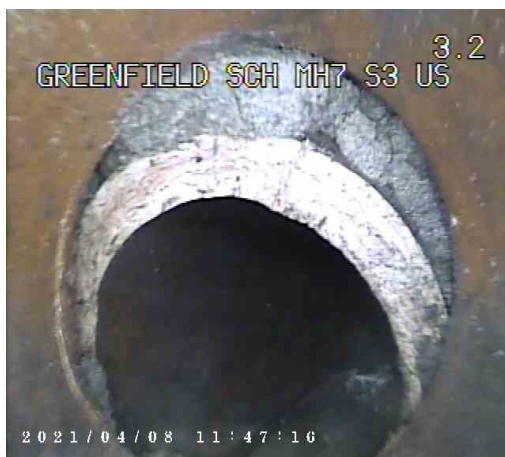
S3X_08081d13-713e-4616-8395-f5720fc488ca_20210409_13 1314_018.jpg, 00:00:21, 3.40 m Joint displaced, large
