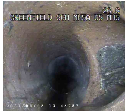
MH5X_3de3c608-3ca9-4df5-82a4-0cbb77bf69d4_20210409_124610_717.jpg, 00:03:28, 26.50 m Junction at 3 o'clock, diameter: 100mm
