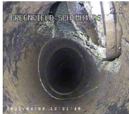
MH4X_c281e691-c5dd-4067-893f-dc45341f6845_20210409_115448_307.jpg, 00:00:26, 2.20 m Connection other than junction at 2 o'clock, diameter: 100mm
