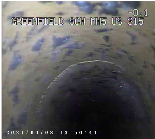
S15X_c113b6bd-6e6c-495a-9882-878ab48ba0b2_20210409_152006_206.jpg, 00:00:11, 0.30 m Crack, circumferential from 9 o'clock to 2 o'clock
