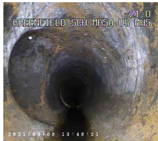
MH5X_bf7cc711-0405-4473-80bf-90adac1f197a_20210409_1 22030_112.jpg, 00:02:52, 20.70 m Junction at 9 o'clock, diameter: 100mm
