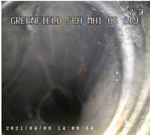
S19X_dd9d0d94-ce81-4efb-9e94-30d3a27859e2_20210409_112824_126.jpg, 00:00:34, 7.50 m Line deviates down
