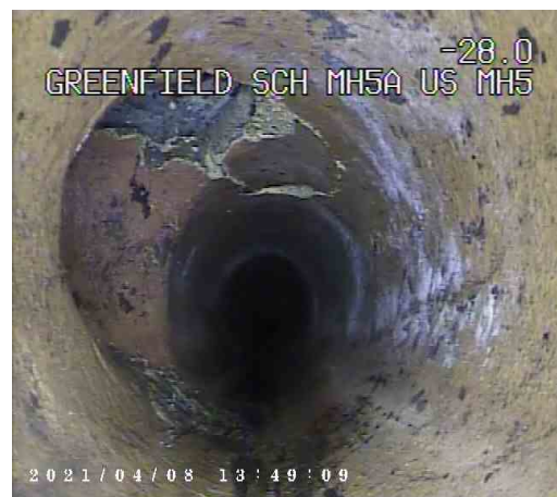
MH5X_3e04c64e-b1fe-4b77-907c-be5f65923622_20210409_124842_293.jpg, 00:03:40, 27.80 m Junction, damaged at 9 o'clock, diameter: 100mm, cracks around junction and surface has broken away at roof of junction.
