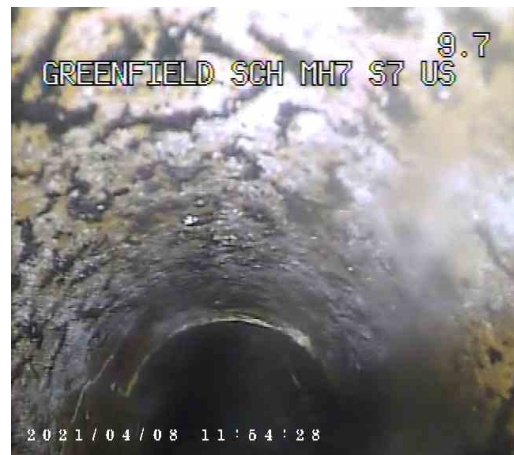
S7X_86844c6d-d3c3-4dae-ae76-a470b62a408f_20210409_133525_000.jpg, 00:00:39, 9.60 m Settled deposits, coarse, 5% cross-sectional area loss, start
