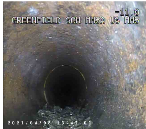
MH5X_384328d5-bbaf-43b1-b6b0-d0c3f9624988_20210409_121516_856.jpg, 00:00:58, 8.30 m Settled deposits, coarse, 10% cross-sectional area loss, start
