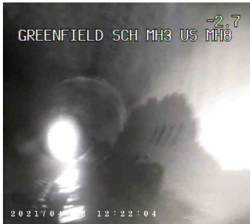
MH8X_2166d7ee-ef24-43fc-8107-9c3dc2aaf9d9_20210409_1 13500_493.jpg, 00:00:22, 2.70 m Water level, 0% of the vertical dimension
