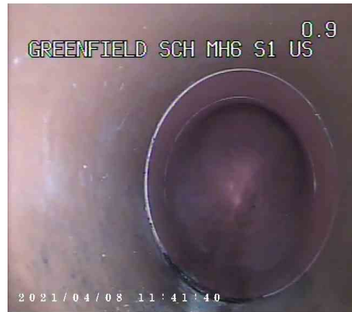
S1X_19ca1c7e-920f-4f7f-a9b8-e17fe0d7bf5c_20210409_1303 25_598.jpg, 00:00:10, 1.00 m Line deviates up
