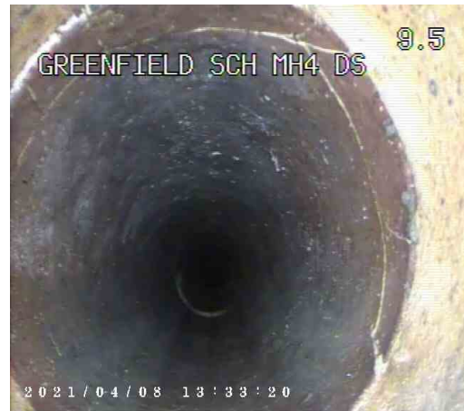
MH4X_5489f68a-388c-47fa-8197-1a58b960e300_20210409_115957_561.jpg, 00:01:58, 9.70 m Crack, circumferential at joint from 9 o'clock to 4 o'clock
