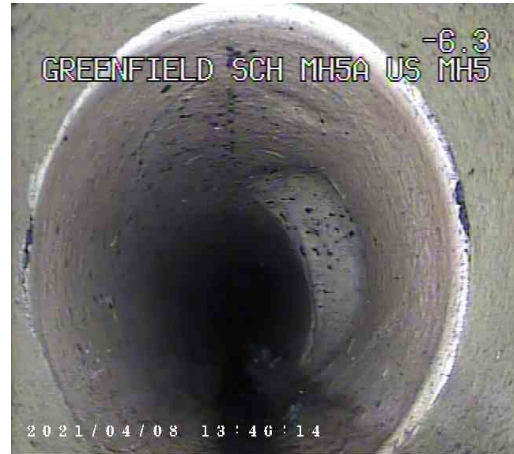
MH5X_f93115d9-cea1-4036-8b8e-14dbf8a3a84a_20210409_120334_338.jpg, 00:00:44, 6.30 m Connection other than junction at 3 o'clock, diameter: 100mm
