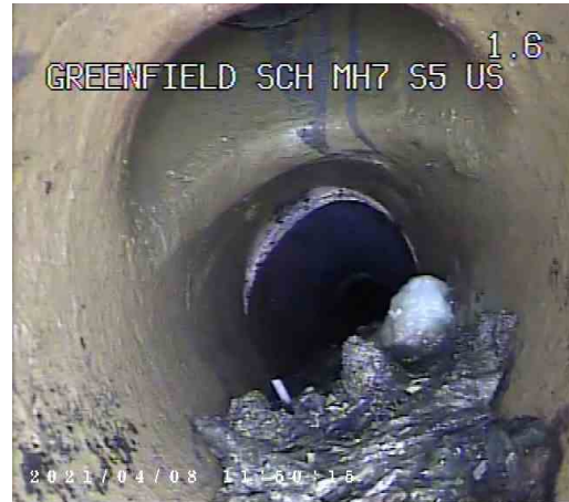
S5X_990815f3-9e2d-435f-86be-476a1ba6b88a_20210409_13 2429_553.jpg, 00:00:11, 1.60 m Settled deposits, coarse, 10% cross-sectional area loss, start
