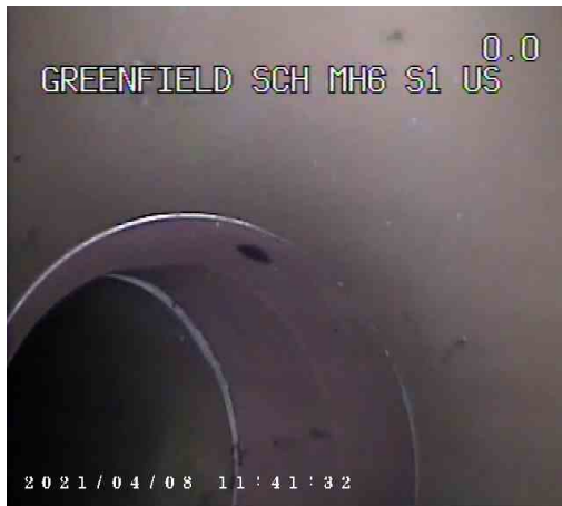
S1X_0ecd798d-34c4-490e-b51f-78300f2b0124_20210409_12 5820_861.jpg, 00:00:02, 0.30 m Line deviates left
