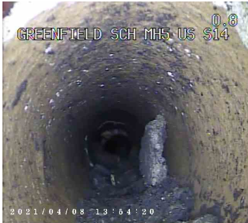
S14X_64b2182a-1397-4ba6-b866-a1851ed92341_20210409_151635_286.jpg, 00:00:06, 0.80 m Settled deposits, coarse, 5% cross-sectional area loss, start
