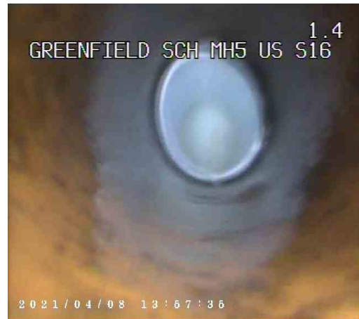
S16X_1de308cd-0bd9-40b1-af55-92919569234e_20210409_ 152236_813.jpg, 00:00:14, 1.40 m Survey abandoned, End of line in building
