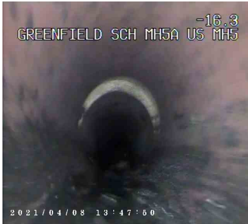
MH5X_7f03486a-89f9-4ab3-bba0-de8f049f1135_20210409_1 21840_128.jpg, 00:02:21, 16.10 m Joint displaced, medium
