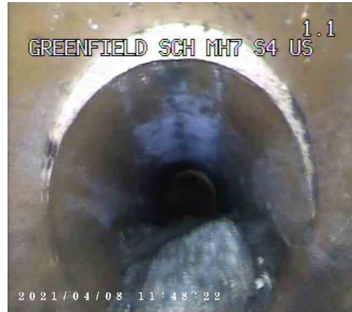
S4X_5506ed63-ef6f-458f-85c2-470b96b1d029_20210409_13 1550_066.jpg, 00:00:08, 1.10 m Settled deposits, coarse, 10% cross-sectional area loss, start
