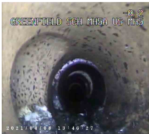
MH5X_d11b7c41-9c04-4916-954e-1ee8bb77c292_20210409_121229_612.jpg, 00:00:58, 8.50 m Junction at 9 o'clock, diameter: 100mm
