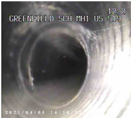
S19X_21fa4948-da78-44f8-b296-5c18644e2fec_20210409_1 13231_501.jpg, 00:01:01, 12.50 m Line deviates right
