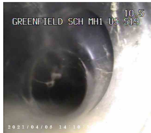
S19X_79bd56e4-7b59-4091-9103-caa22f5ceb1d_20210409_113137_271.jpg, 00:00:51, 10.75 m Junction at 3 o'clock, diameter: 150mm
