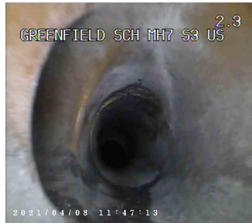
S3X_e2d87558-950d-4720-a65b-363b13c3e288_20210409_1 31250_314.jpg, 00:00:18, 2.40 m Junction at 9 o'clock, diameter: 100mm
