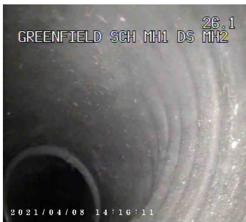
MH1X_80bbb0b6-74e0-48e5-8f15-96d0218fb9a5_20210409_110136_624.jpg, 00:03:08, 26.10 m Line deviates down
