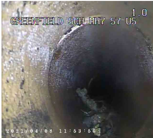
S7X_59a4078a-df71-4787-89bc-8338e67859ba_20210409_133206_000.jpg, 00:00:07, 0.80 m Settled deposits, coarse, 5% cross-sectional area loss, start
