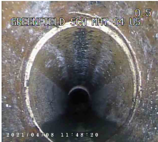
S4X_633130cf-93ca-4fc3-9c14-b2304613b7c7_20210409_13 1515_171.jpg, 00:00:05, 0.67 m Crack, circumferential at joint from 12 o'clock to 12 o'clock
