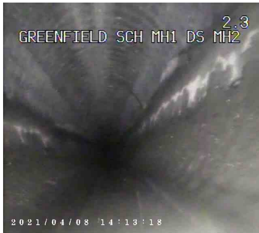
MH1X_f96da183-a2df-487f-bae7-30318694c6ec_20210409_1 05429_003.jpg, 00:00:13, 1.90 m Water level, 5% of the vertical dimension
