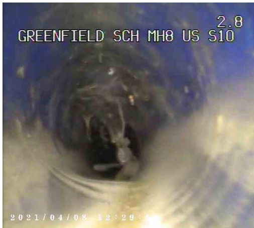
S10X_a237a71e-862e-4f3e-aa15-d3d8db956608_20210409_134349_695.jpg, 00:00:15, 3.00 m Deformed sewer or drain, 5%, Floor of pipe pushed in.
