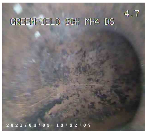
MH4X_898e3ae4-a4e6-42f0-a37a-9054f851f5dc_20210409_115725_890.jpg, 00:00:44, 4.80 m Line deviates right
