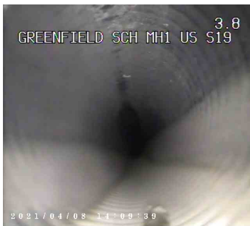
S19X_7ea72eda-0da7-4549-95e6-02b0c66ac28d_20210409_112715_862.jpg, 00:00:18, 3.80 m Water level, 0% of the vertical dimension
