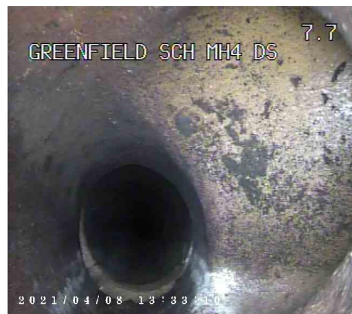
MH4X_1121c319-d81f-439c-b0c2-1f6b5c487b0b_20210409_115848_979.jpg, 00:01:47, 7.80 m Junction at 3 o'clock, diameter: 100mm
