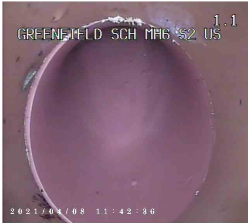
S2X_7fb62b8d-49c5-448e-b280-f56655060e90_20210409_13 0642_195.jpg, 00:00:13, 1.20 m Line deviates up
