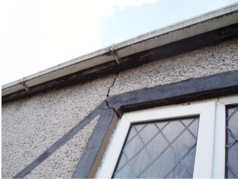
The large crack above the window
