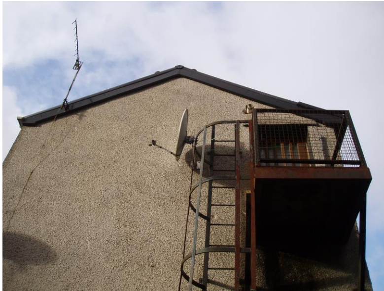
Eastern facing gable, gaps beneath UPVC fascia
