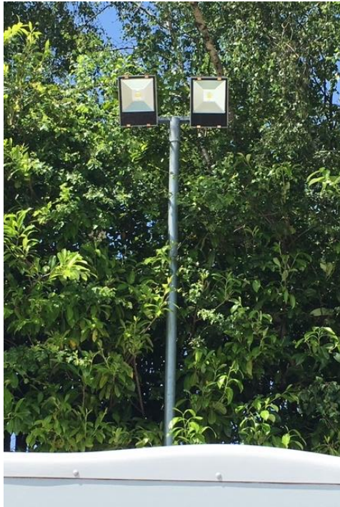
1. Existing lighting column
