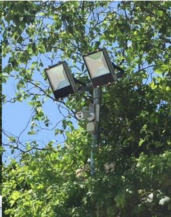
2. Close up of flood lights
