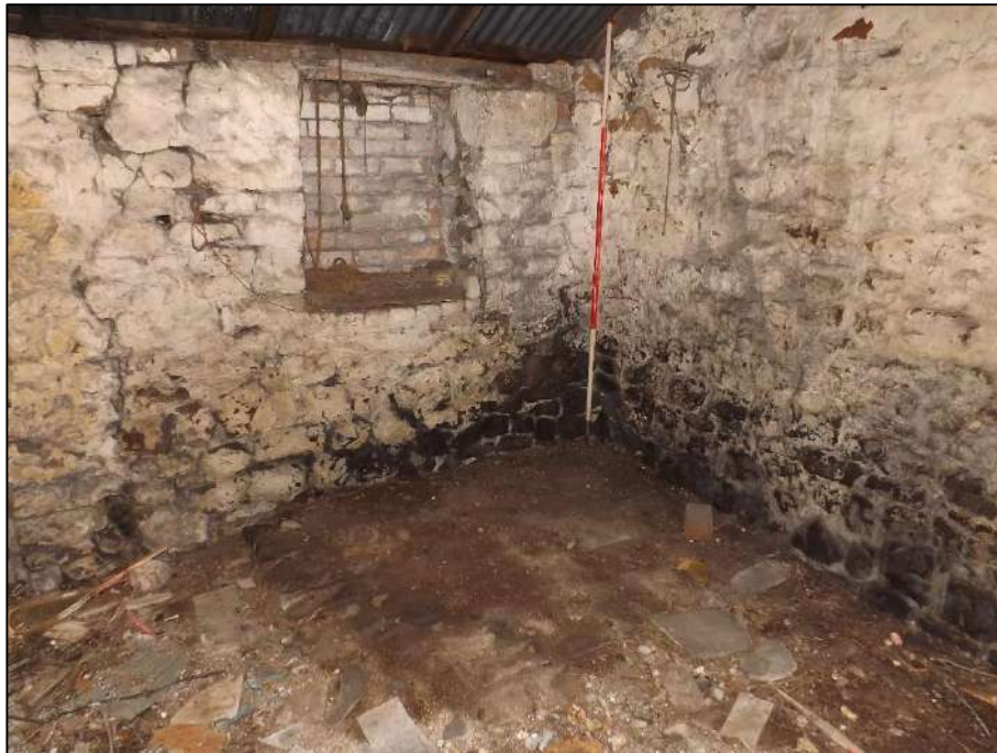
Plate 16. North west corner of Annexe 1 showing the blocked window and raised floor. Just visible is the modern corrugated iron roof. Scale 2m.
