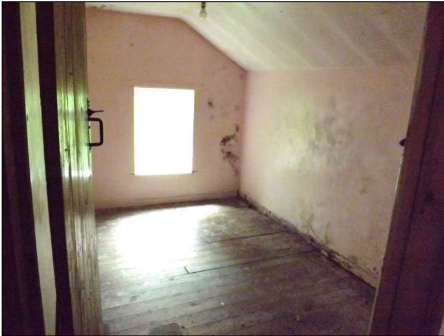
Plate 44. View into the north west bedroom. Rotten floorboards prevented entry into the room.
