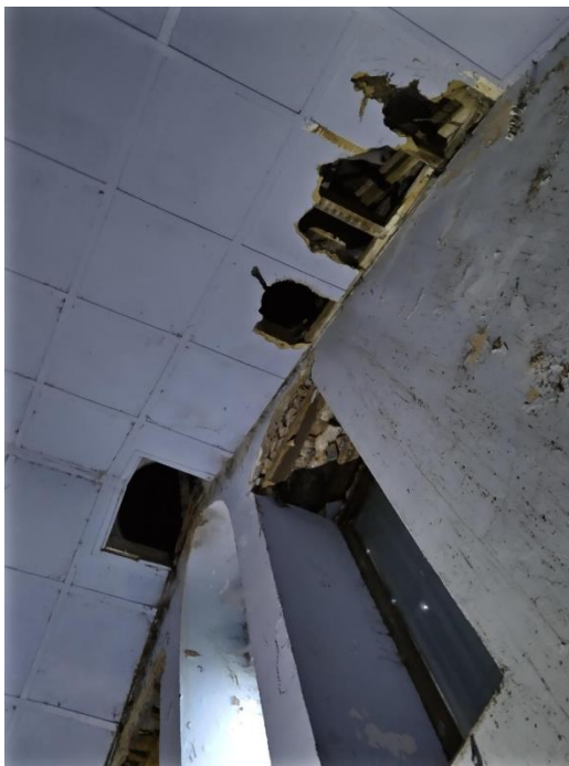
Figure 24 - Gaps in the ceiling on the second floor.
