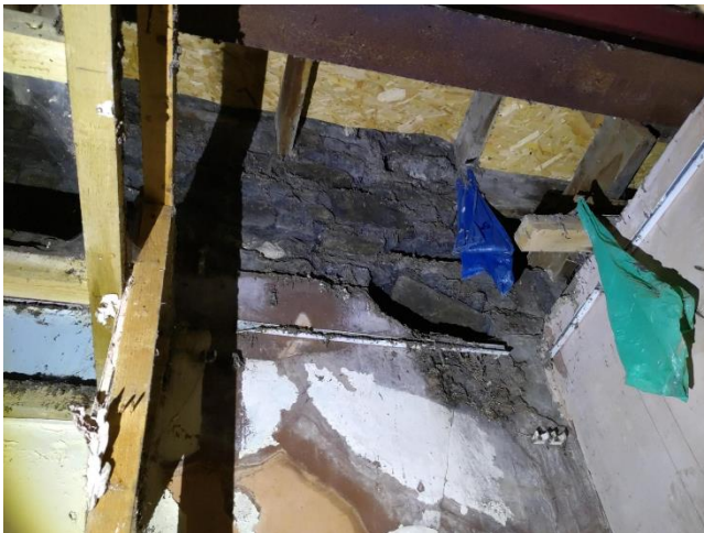
Figure 20 - Gaps in brickwork on first floor.
