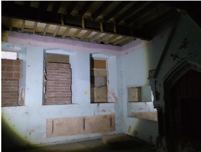
Figure 10 - Bricked up windows on the ground floor.
