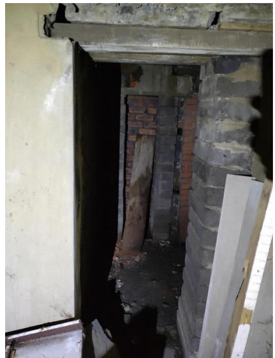
Figure 33 - Gaps in brickwork in northern basement.
