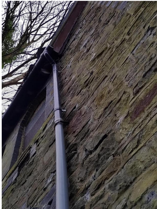
Figure 38 - Gap between wooden soffit and wall on northern aspect of the building.
