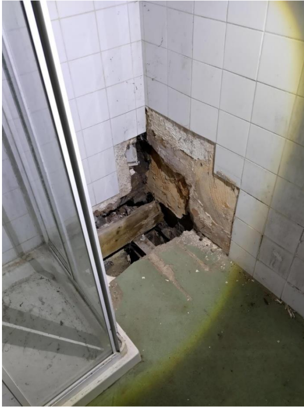
Figure 18 - Hole in shower room floor on ground floor leading to basement.
