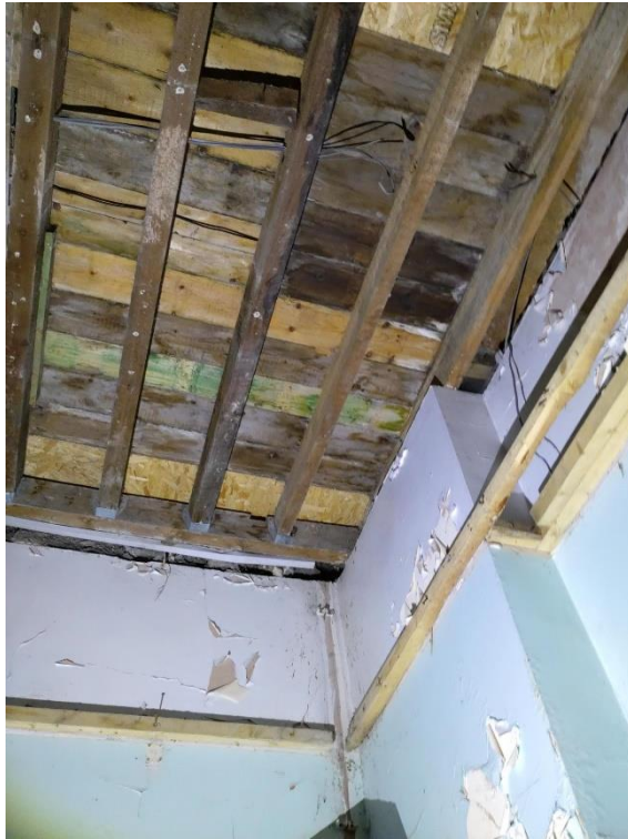
Figure 14 - Gaps between walls and ceiling on ground floor.
