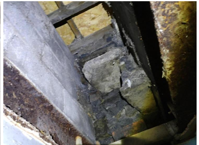
Figure 214 - Gaps in stonework on first floor.
