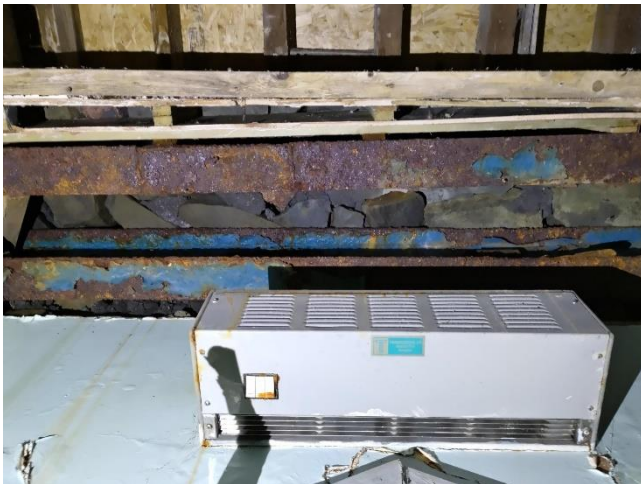
Figure 12 - Gaps in stonework in roof of ground floor.
