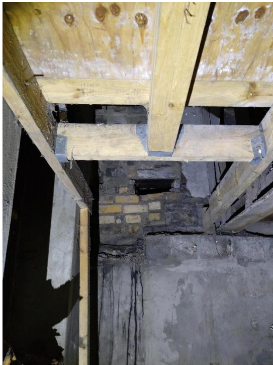
Figure 32 - Gaps in brickwork in northern basement.
