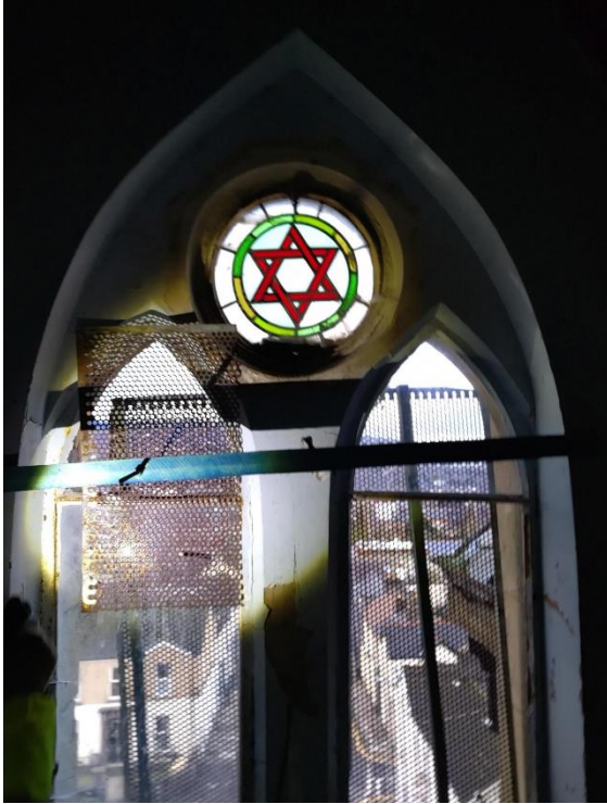
Figure 26 - Gaps in window on second floor.
