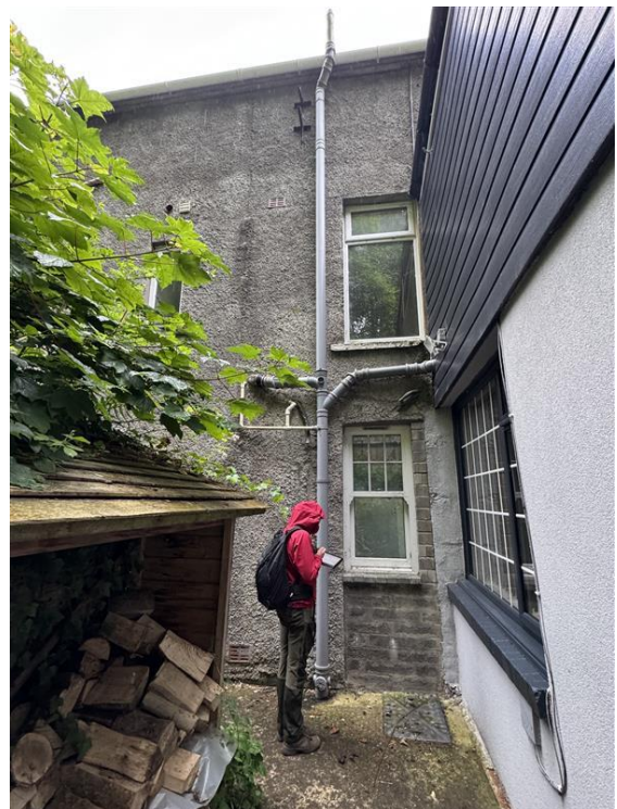
Figure 49 - North-west corner of Primrose Hill (with ground floor window to be changed to door).
