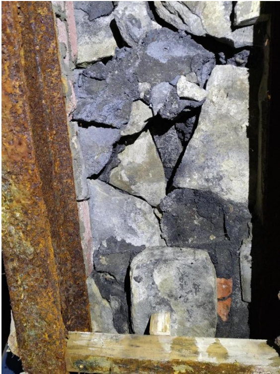
Figure 34 - Gaps in brickwork in northern basement.
