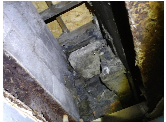
Figure 13 - Gaps in stonework in roof of ground floor.
