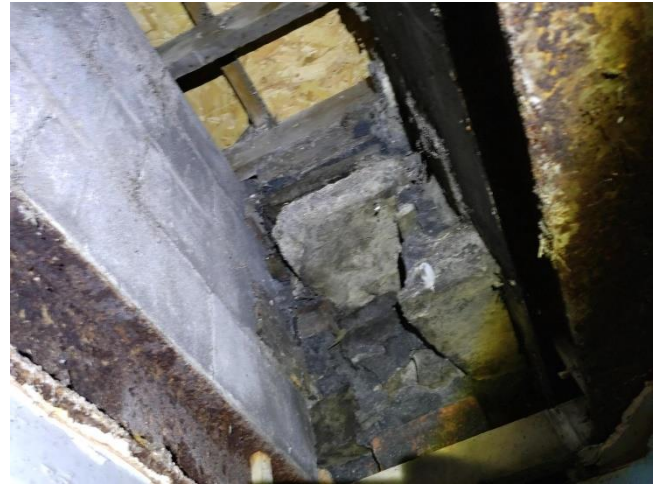
Figure 214 - Gaps in stonework on first floor.
