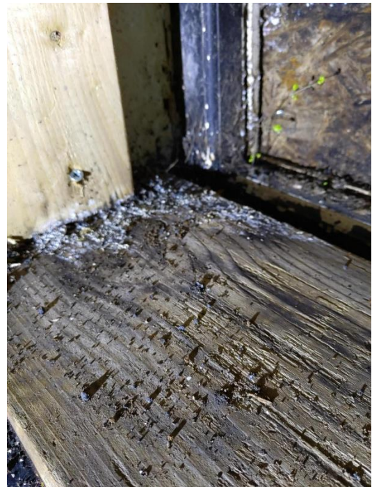
Figure 17 - Bird droppings on a windowsill on the ground floor.
