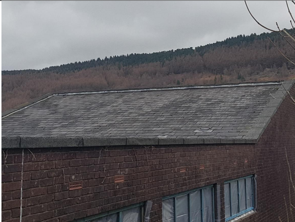
Photo 8 Slate mono- pitch with some misalign ed slates
