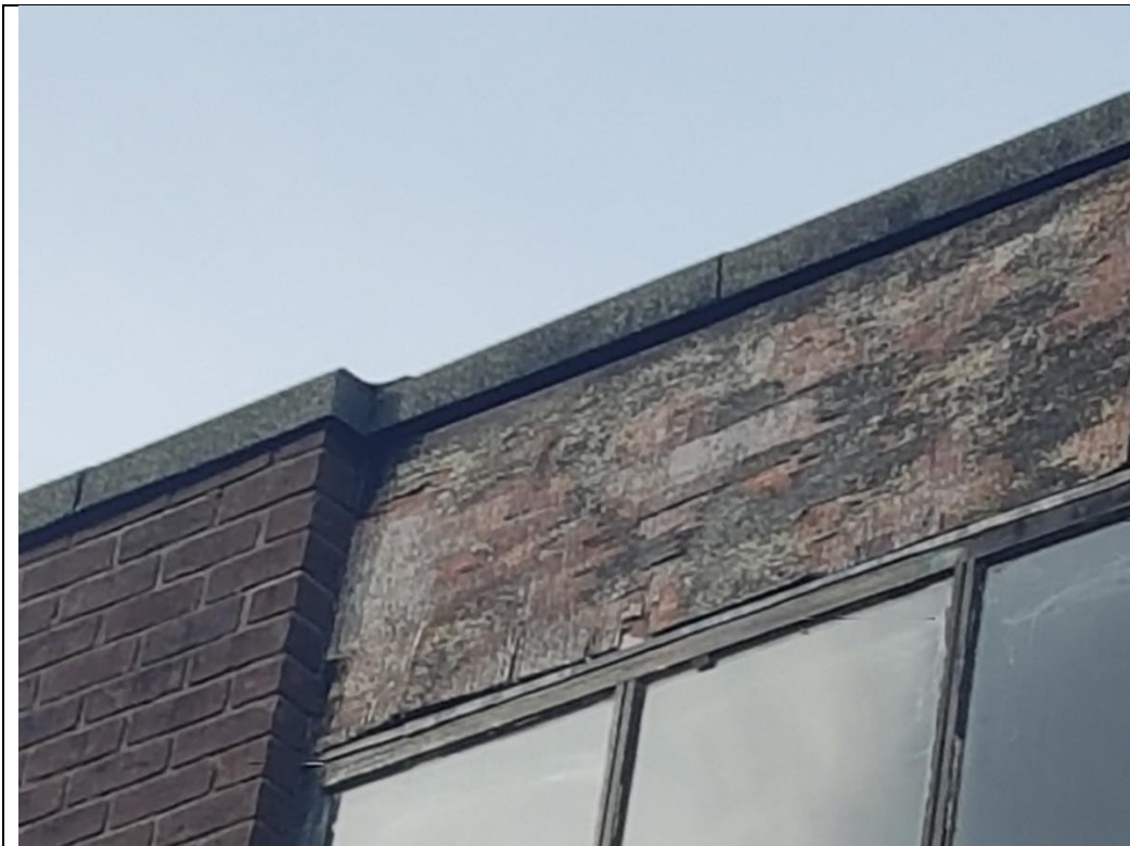
Photo 5. Gaps in boarding to east
