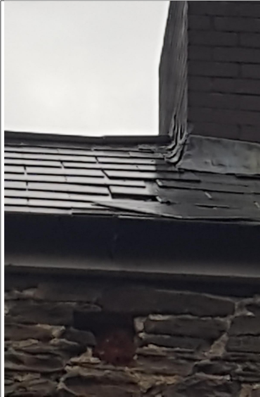
Photo 6. Gaps at chimney flashing and misalign ed slates
