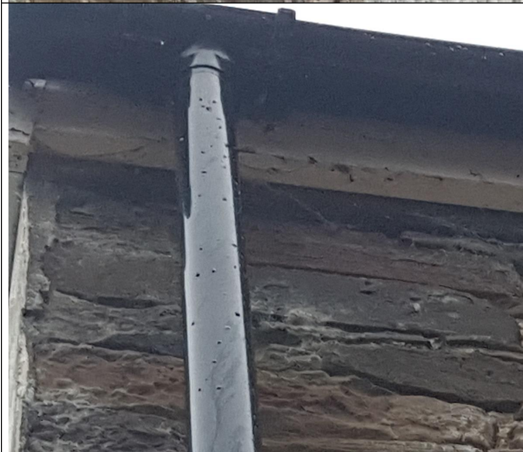
Photo 5. Gaps at the rear fascia
