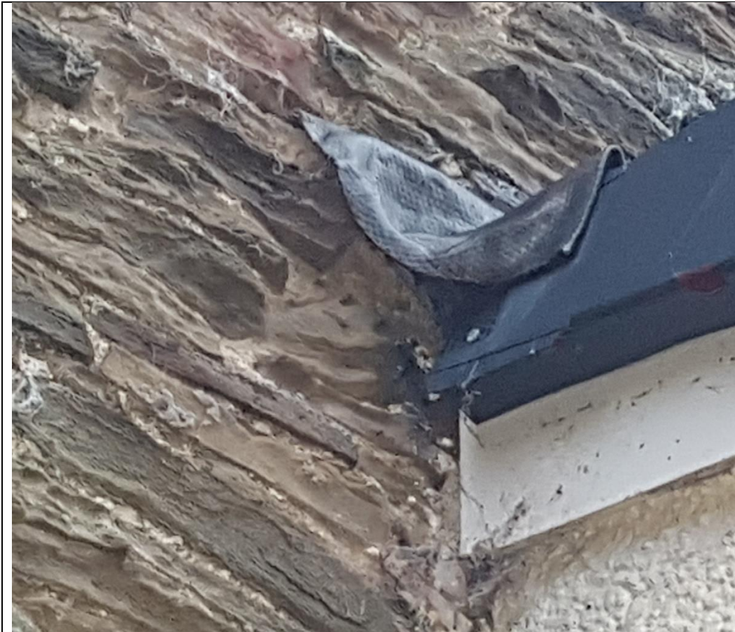
Photo 4. Gap at the flashing extensio n at roof tie- in
