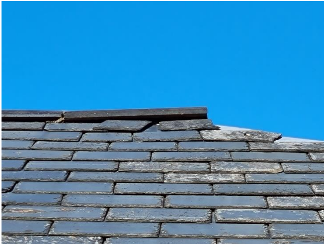
Figure 9 – Frequent slipped/missing tiles.
