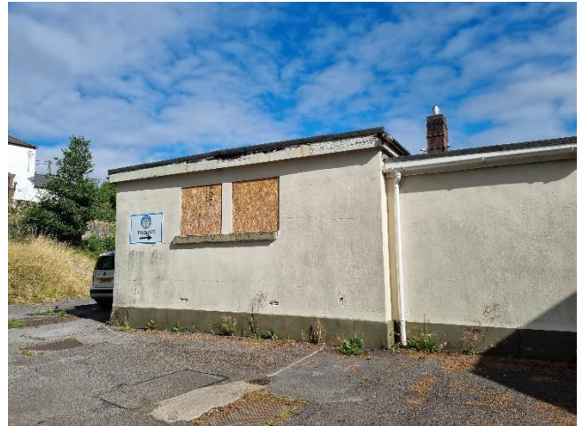
Figure 10 – South-western corner of building, showing rotting timbers under flat roof.
