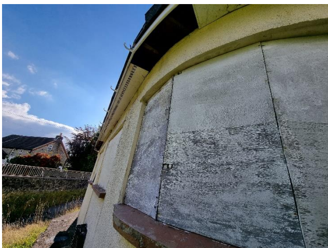
Figure 15 - Small building at south-west of site with gaps in soffit.
