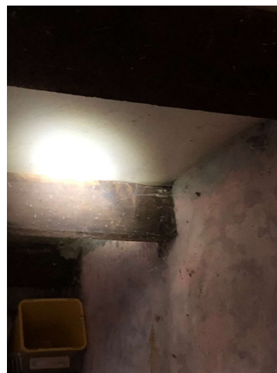
Figure 3 Internal beam of garage showing crevice between ceiling
