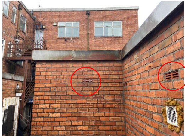
Photo 8: Example of Vents on the Single-storey Extensions
