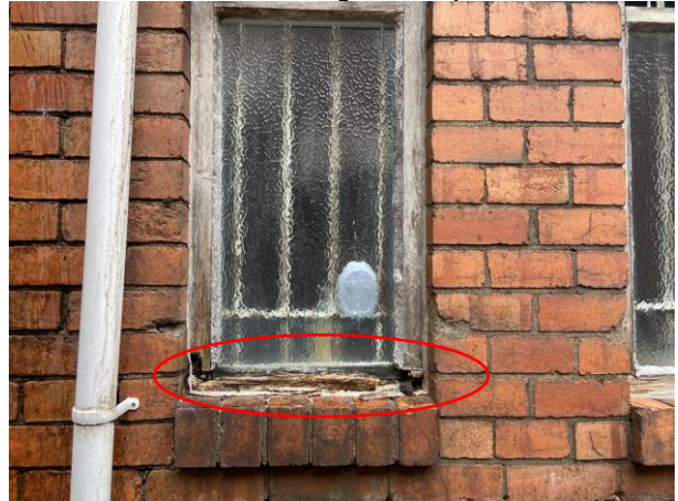
Photo 10: Rotten Window Frame (Circled) on Southern Elevation of Single-storey Extension
