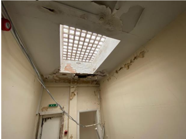
Photo 5: Internal View Showing Stairwell Open to the Ceiling
