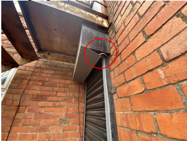
Photo 11: Roller Shutter Door With Metal Frame Showing Large Gap (Circled)
