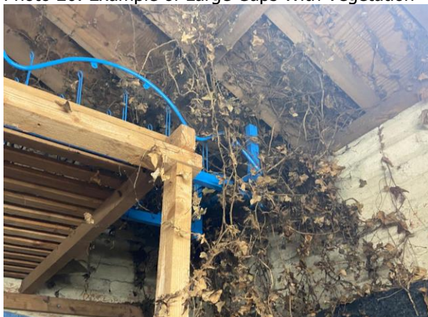
Photo 26: Example of Large Gaps With Vegetation
