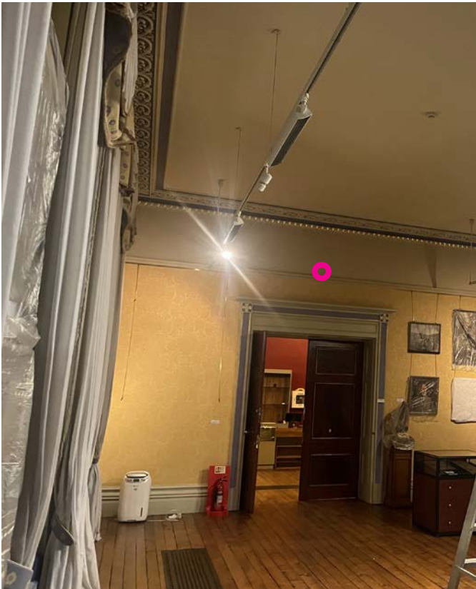
New camera locations above doors and above picture rail to get full coverage of the room. Cabling route not visible above picture rail
