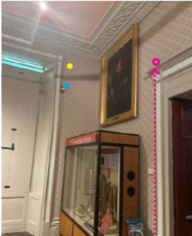
Trunking to be wrapped in wallpaper to match wall
