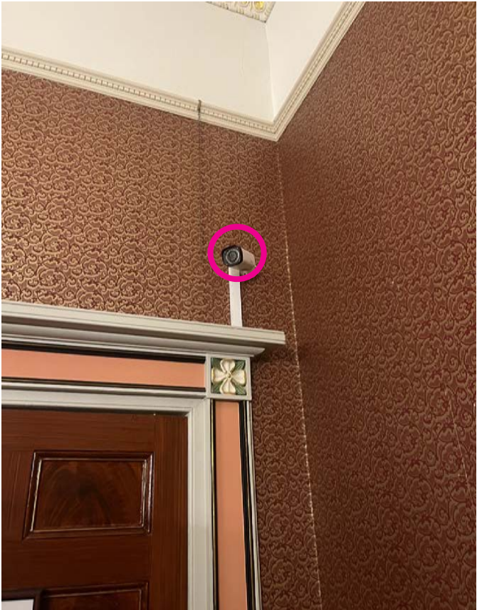
Trunking to be wrapped in wallpaper to match wall
