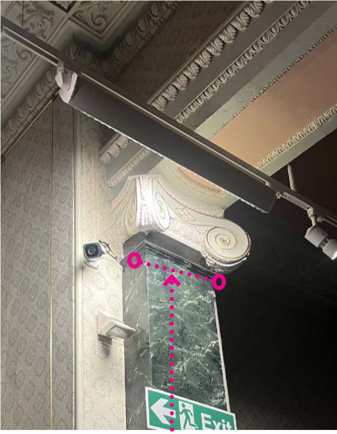
F2 & F3 - New drilled hole in pilaster will be required hidden behind camera.
