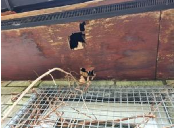
Photo 12: Damaged Timber Soffit Box
