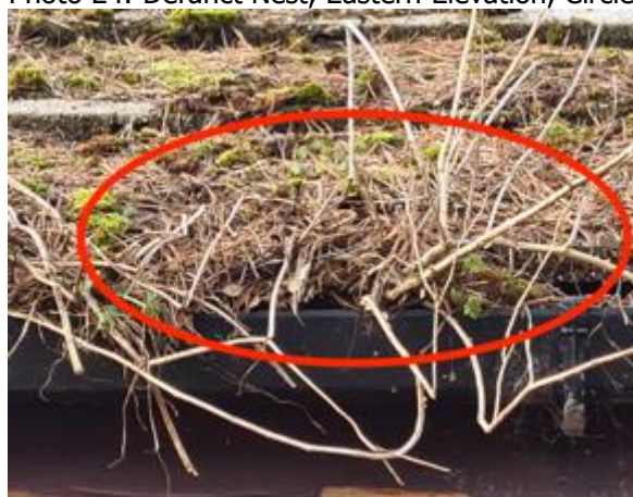
Photo 24: Defunct Nest, Eastern Elevation, Circled
