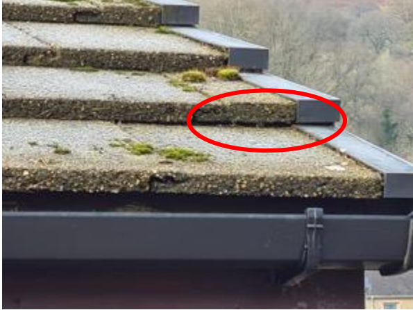
Photo 7: Eastern Elevation Lifted Roof Tile, Circled
