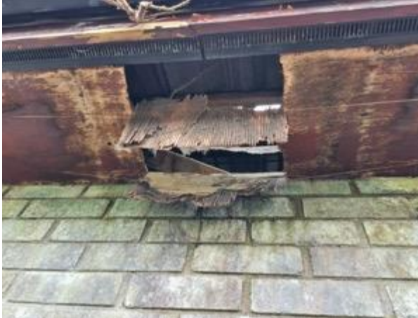
Photo 11: Broken Timber Soffit Box
