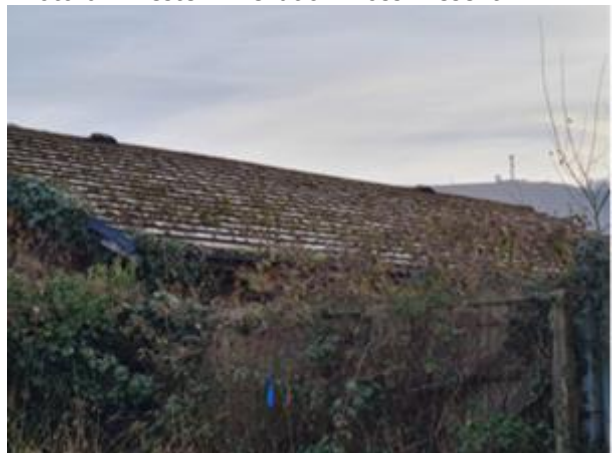
Photo 6: Western Elevation Moss Present
