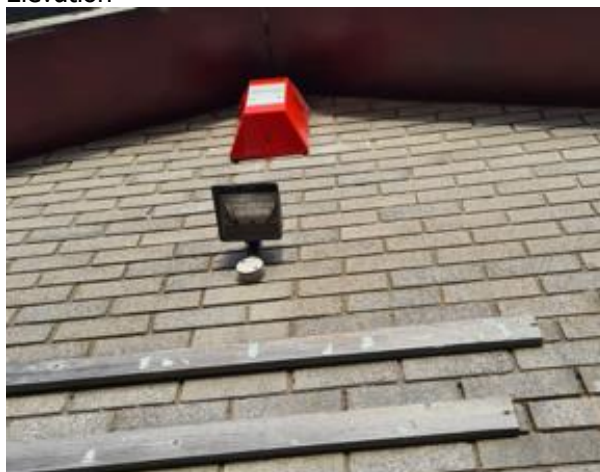
Photo 20: Smashed Security Light, on Southern Elevation
