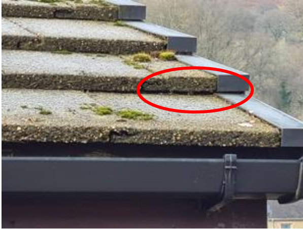
Photo 7: Eastern Elevation Lifted Roof Tile, Circled
