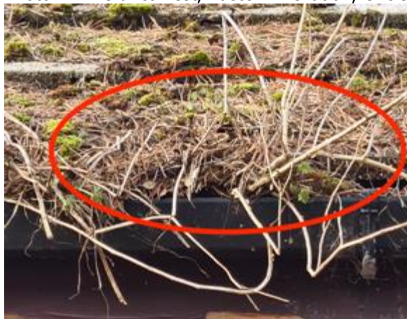
Photo 24: Defunct Nest, Eastern Elevation, Circled
