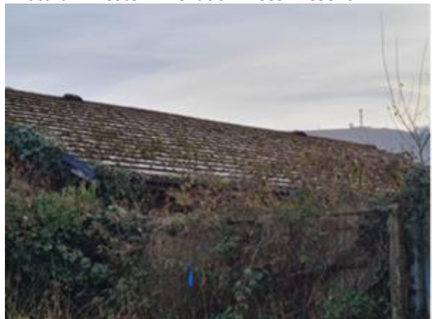
Photo 6: Western Elevation Moss Present
