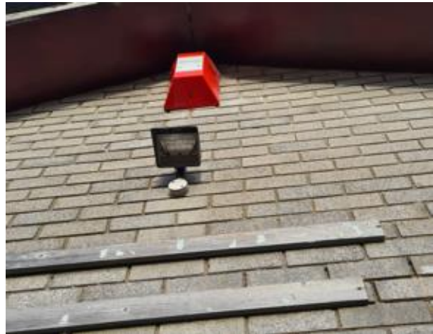
Photo 20: Smashed Security Light, on Southern Elevation
