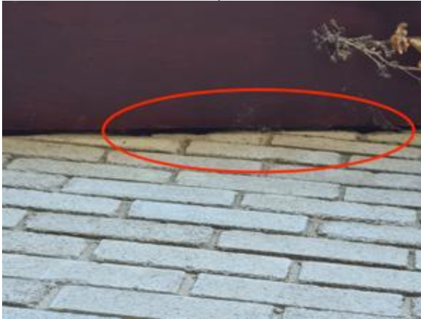
Photo 9: Lifted Timber Soffit Box from Brick Wall on the Southern Elevation, Circled
