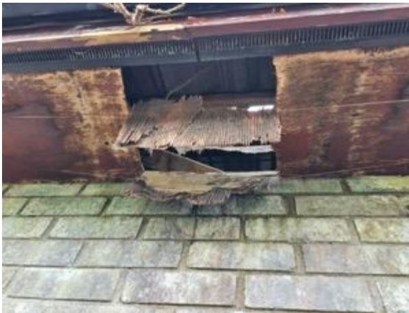
Photo 11: Broken Timber Soffit Box
