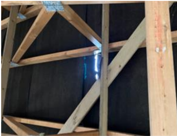
Photo 19: Tear in Bitumen Felt Roof Lining
