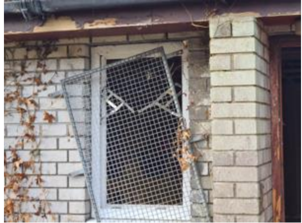
Photo 14: Loose Window Grate
