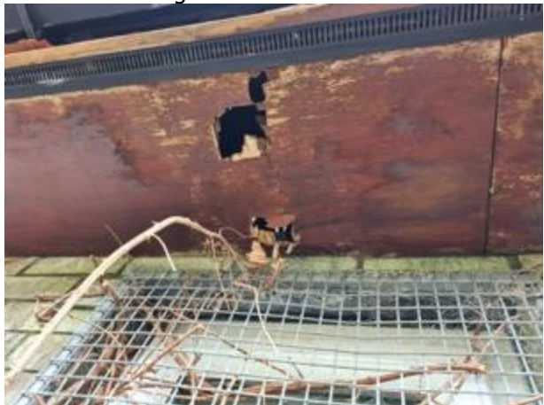
Photo 12: Damaged Timber Soffit Box
