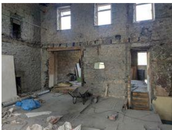
PRF – Internal, upper-floors. Cavities in stonework.
