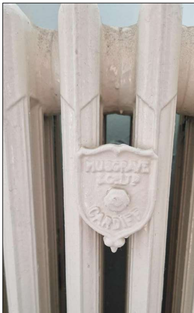
Plate 31. Shield plaque on radiator.
