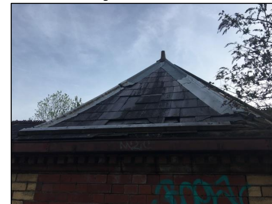
Photo 20 Missing tiles on eastern elevation
