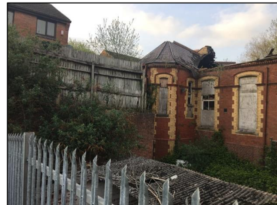
Photo 18 Missing tiles on western elevation
