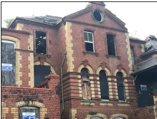
Photo 17 Missing tiles on southern elevation
