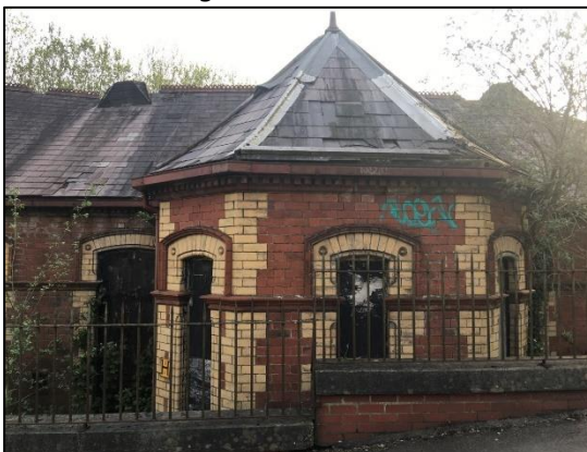
Photo 29 Missing tiles on eastern elevation
