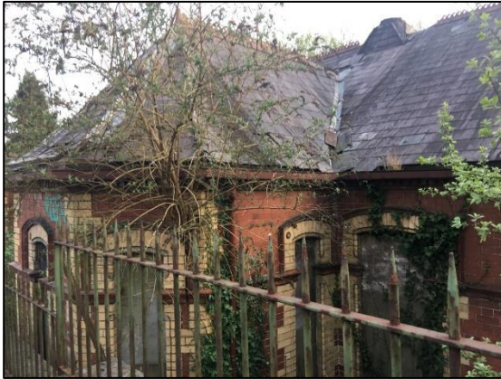
Photo 21 Missing tiles on eastern elevation
