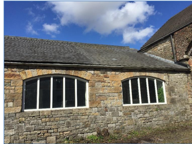
Photograph 14. Building C, northern half of the eastern elevation, with missing ridge tiles and bowing of roof visible.
