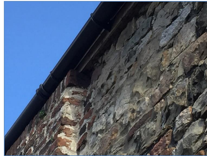
Photograph 8. Building B, eastern section. Further gaps beneath fascia boards.
