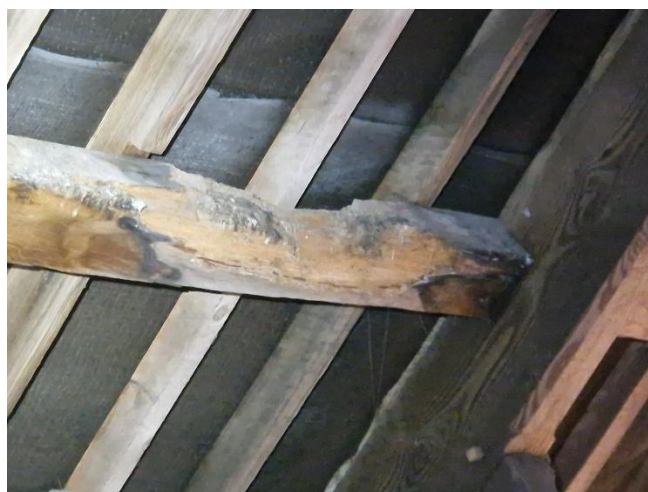
Bay B, South, P2 – decayed section of purlin
