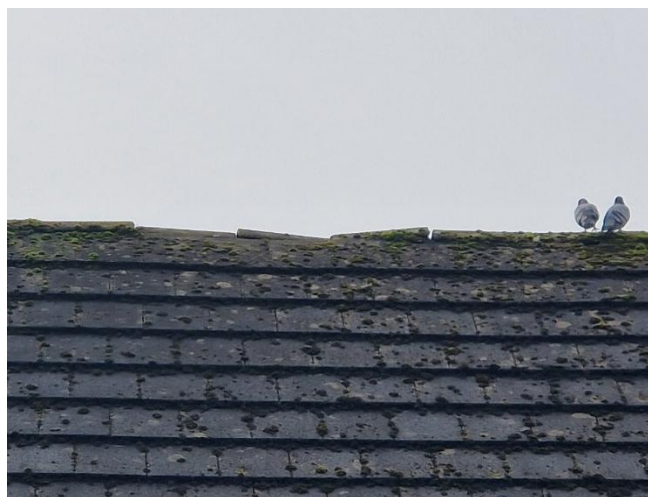
Failed ridge tiles over Bay D
