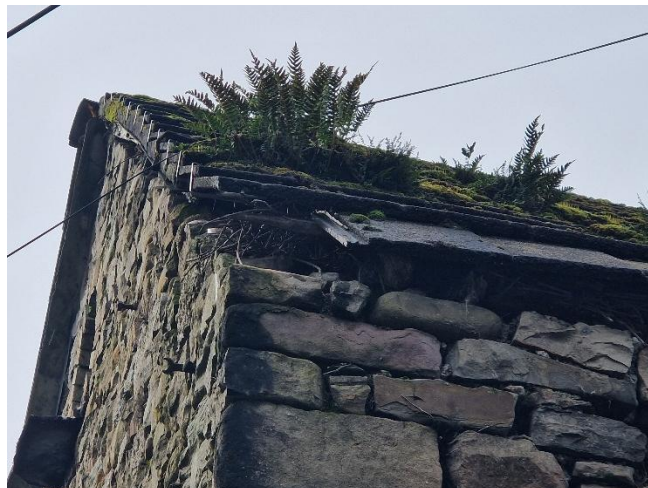
East gable eaves failure
