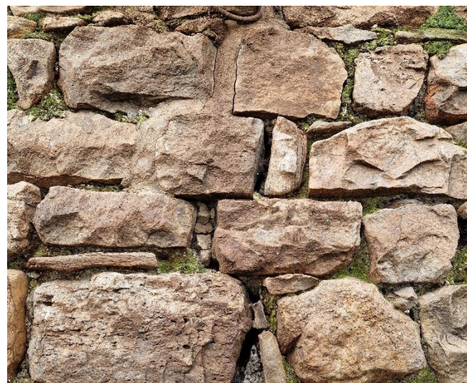
Previous repairs to crack
