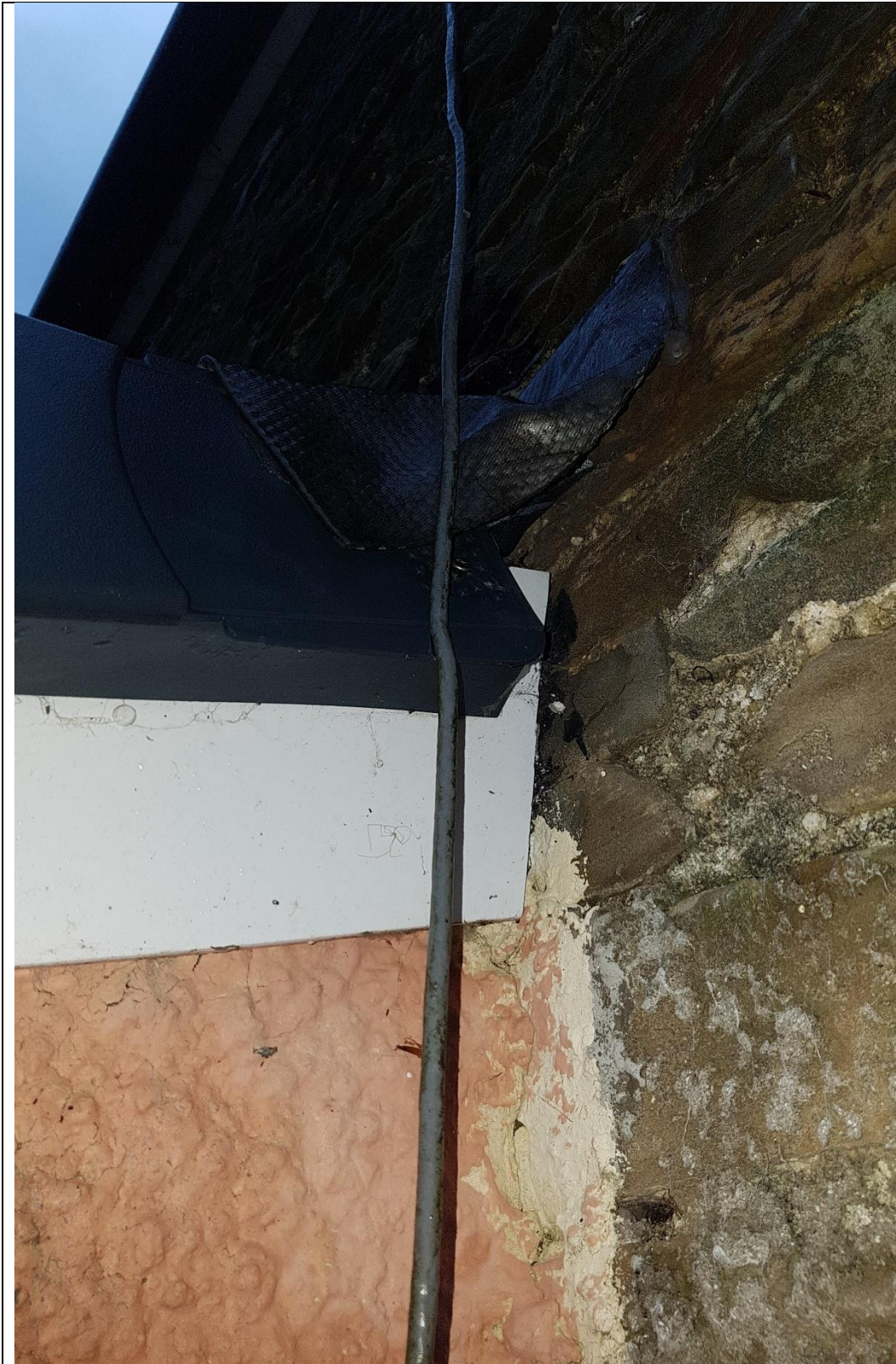
Photo 7. Gaps in flashing edge of extensio n tie-in
