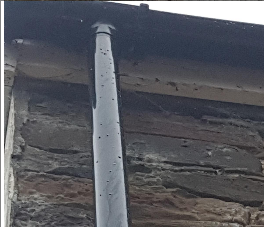
Photo 5. Gaps at the rear fascia
