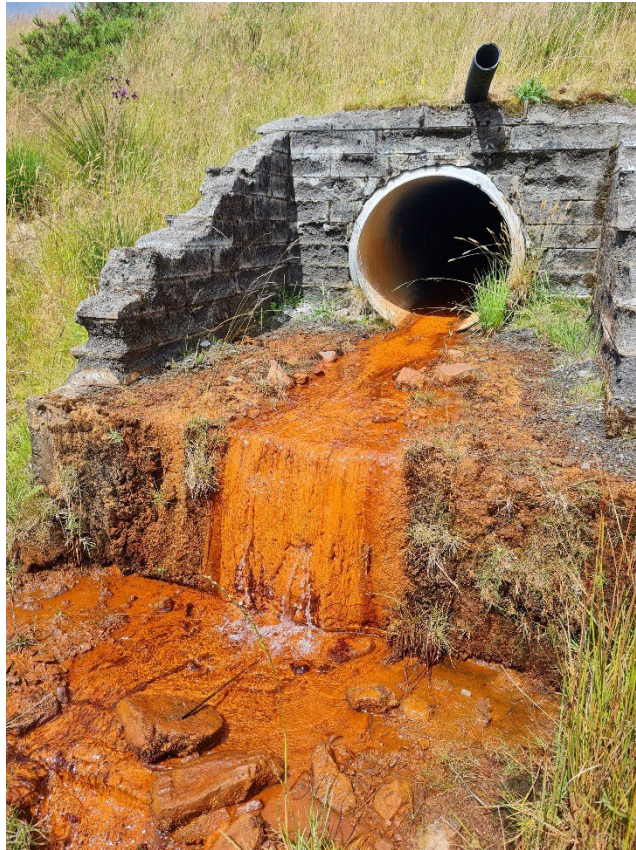
Figure 11 Culvert with orange staining
