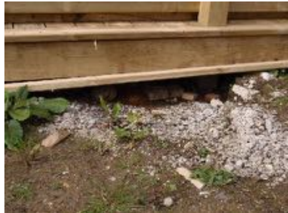
Gap under north west boundary fence
