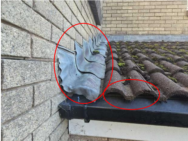
Photo 9: Lifted led flashing and missing wildlife spikes
