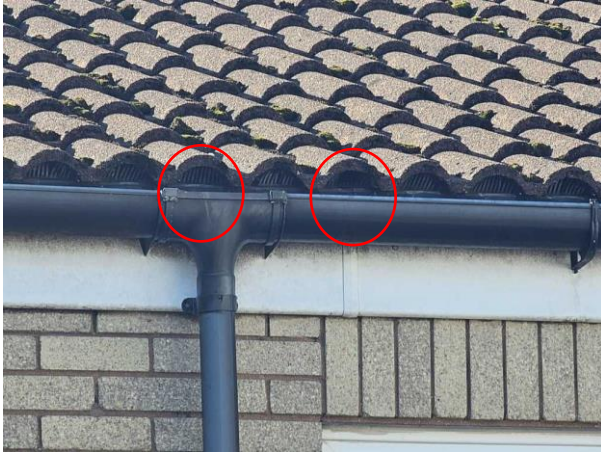
Photo 7: Interlocking tiles with missing wildlife spikes
