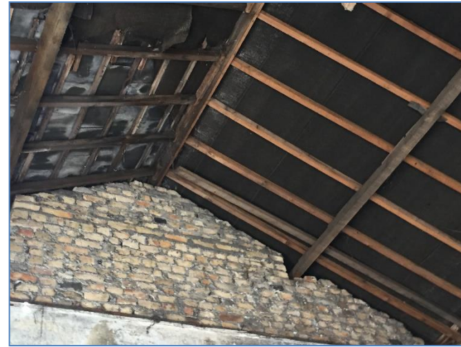
Photograph 30. Building F. Gappy internal wall tops allowing access between sections.
