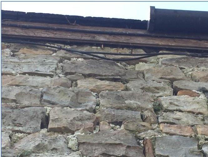
Photograph 7. Building B, eastern section. Gaps beneath fascia boards on the northern elevation.
