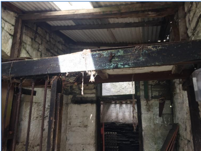
Photograph 19. Building D. The store rooms in a very poor state of repair.
