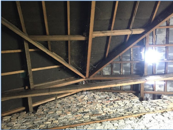
Photograph 31. Building F. Bitumen felt present on most of the western hip.
