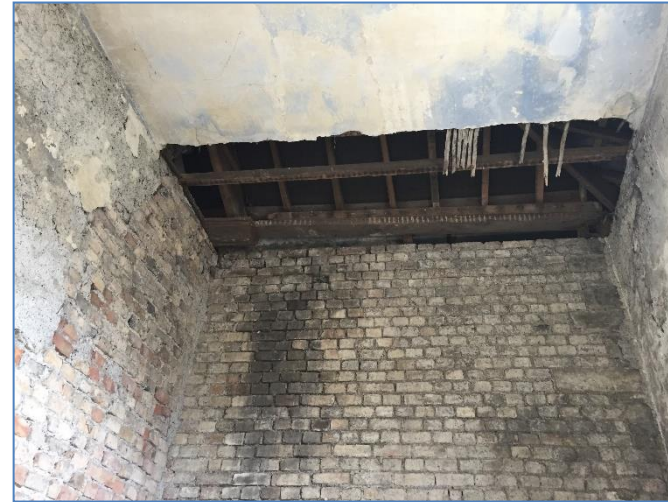
Photograph 32. Building F. A damaged ceiling showing loft space on the eastern end.
