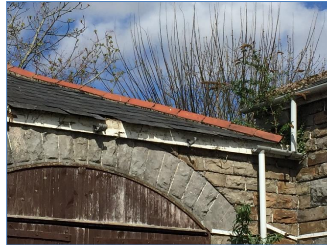
Photograph 22. Building E. Missing tiles from the lower courses.
