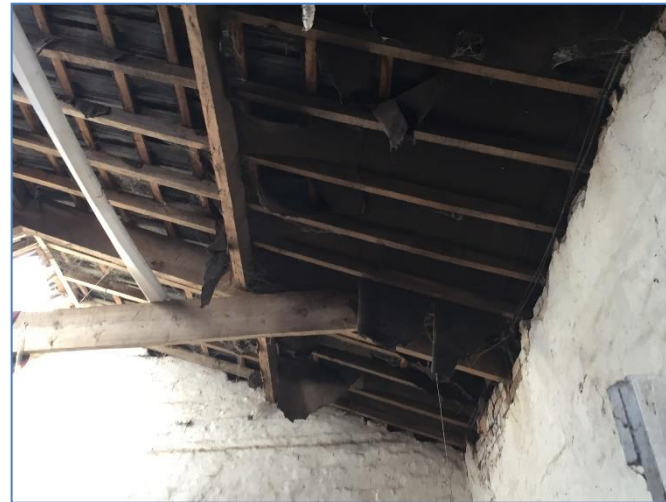
Photograph 40. Building H. Gappy brickwork visible at the wall tops.
