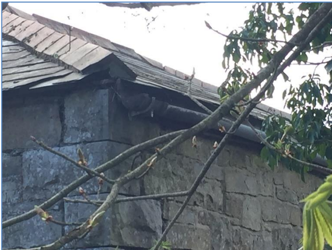
Photograph 23. Building E. The Missing mortar from the hip.
