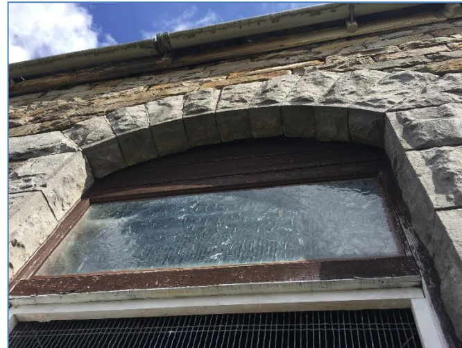
Photograph 28. Building F. Gaps present below window arches.
