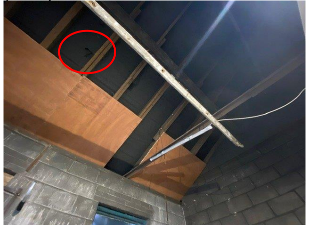
Photo 12: Tear in Roofing Felt of Main Section (Circled)
