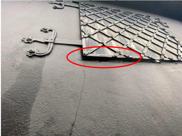
Photo 11: Example of Gaps Between Metal Window Guard and Exterior Wall (Circled)
