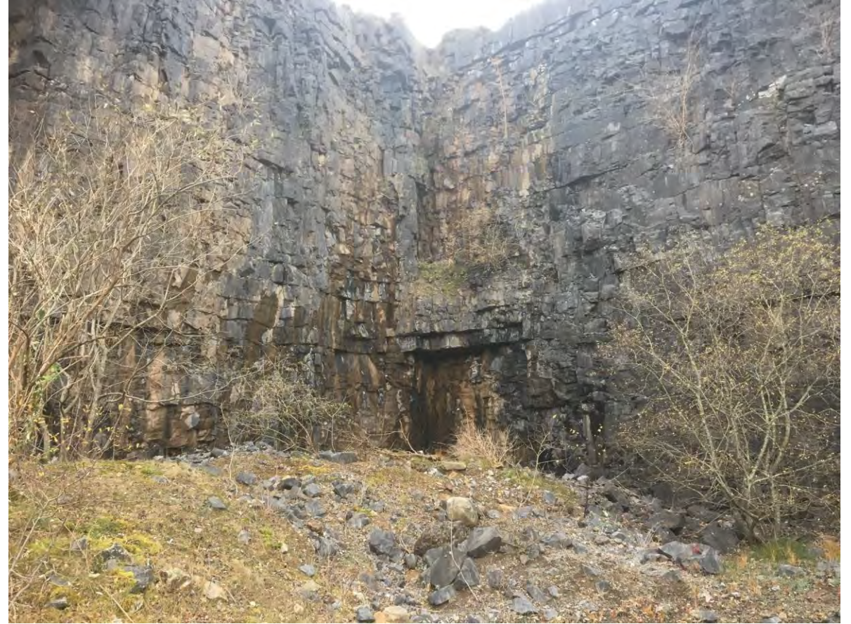
P035 – seepages in north-western corner of eastern arm
