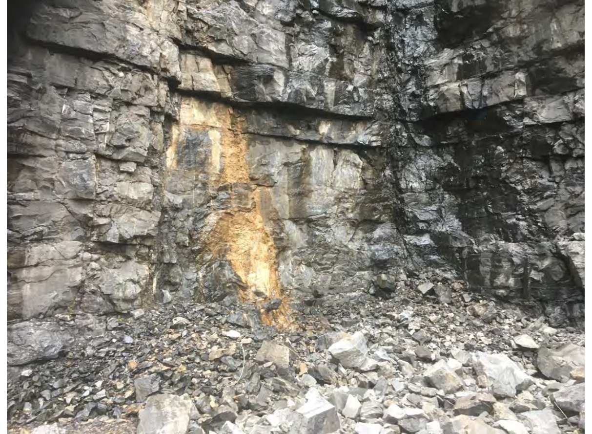
P012 – seepage in NE of lower bench
