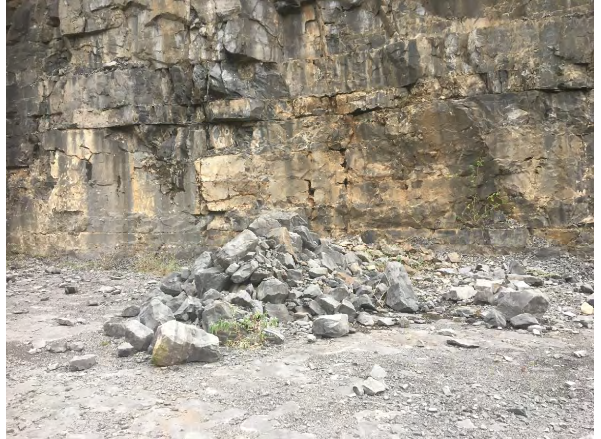
P026 – staining of walls, possibly related to seepages not flowing
