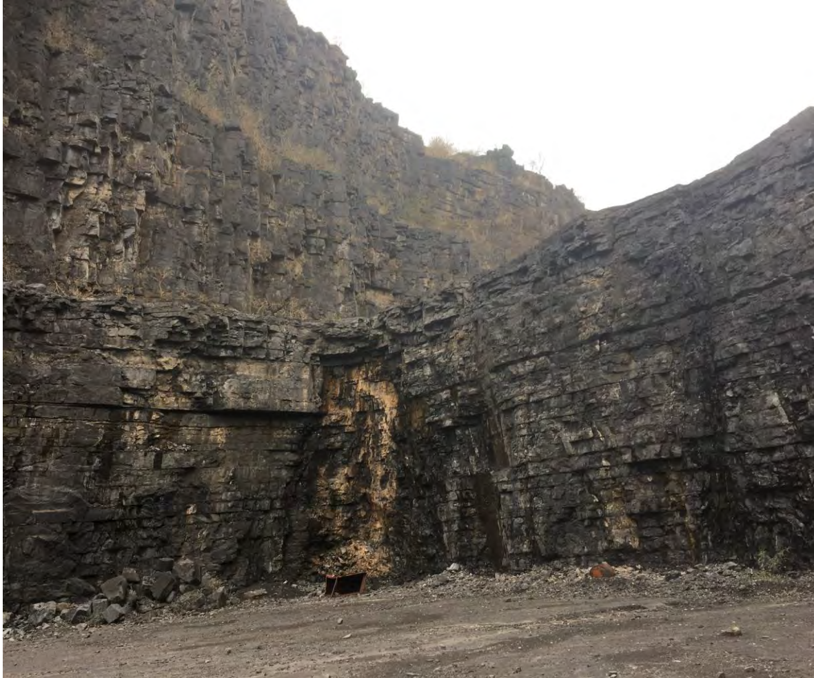
P011 – extensive seepage in NW of lower bench
