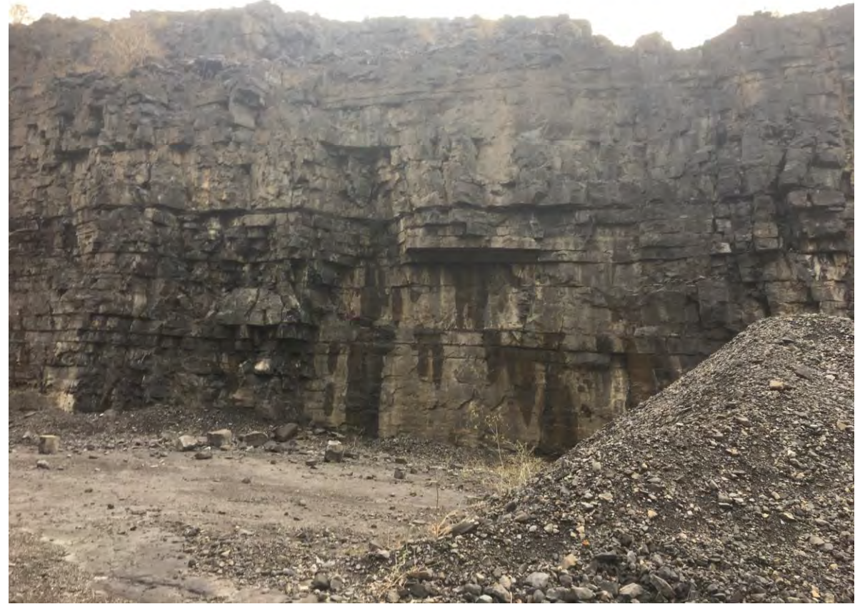
P006 – Seepages along lower face
