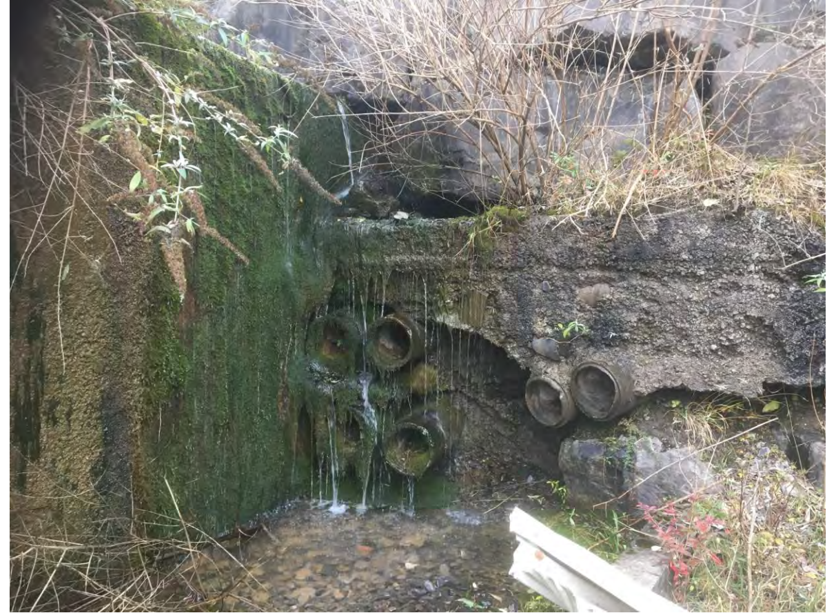
P087 – flow of water towards culvert, water mostly flowing around and not through the pipes
