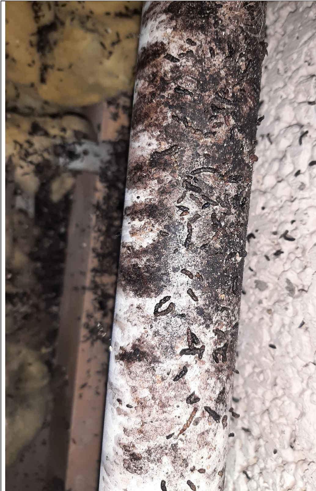
Photo 16. Close up of bat droppings on top of small heater (switched on at time of survey)
