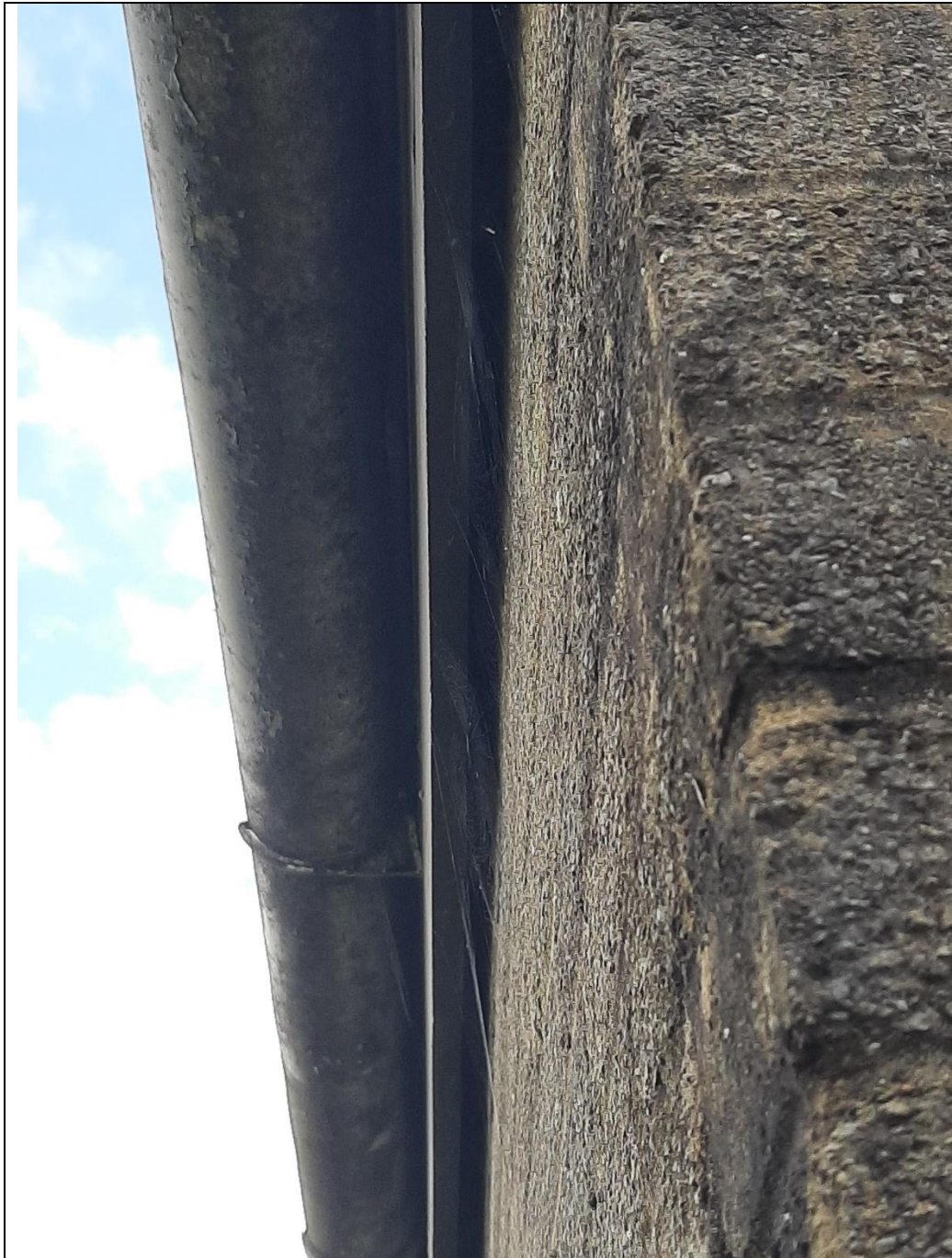
Photo 14. Changing room building gap behind both fascias
