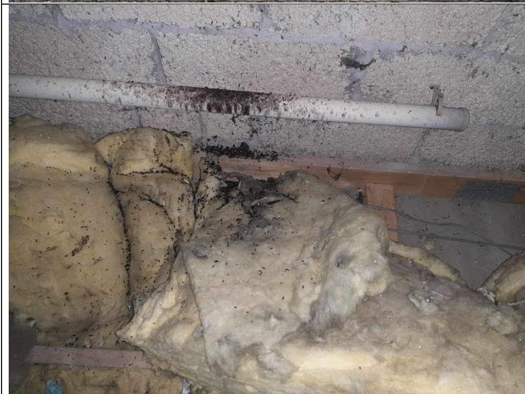
Photo 15. Bat droppings which have fallen into the loft
