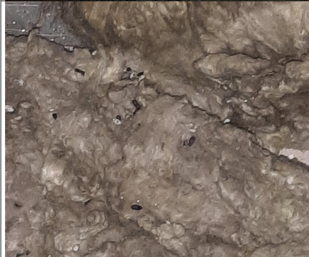
Photo 8 Club house building loft – rodent droppings
