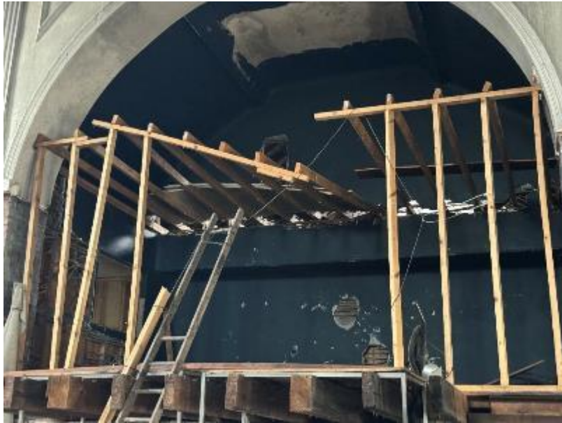
Photograph 18: Failed timber stud framing (Note: multiple loose boards at ceiling level)
