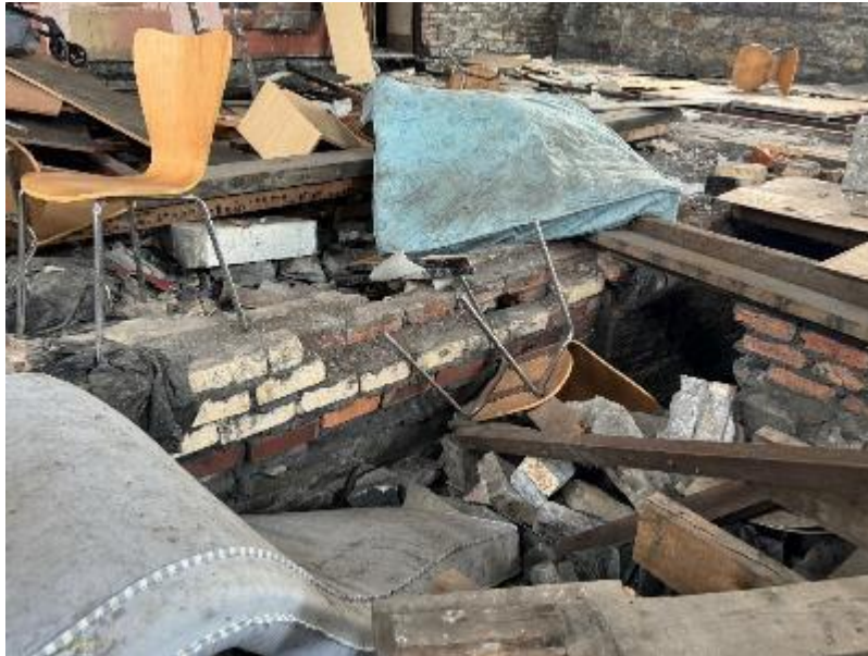
Photograph 24: Damaged and defective masonry local to the basement
