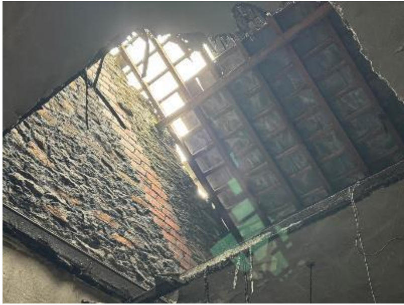
Photograph 7: Defective ceiling / roof structure (Rear Extension)
