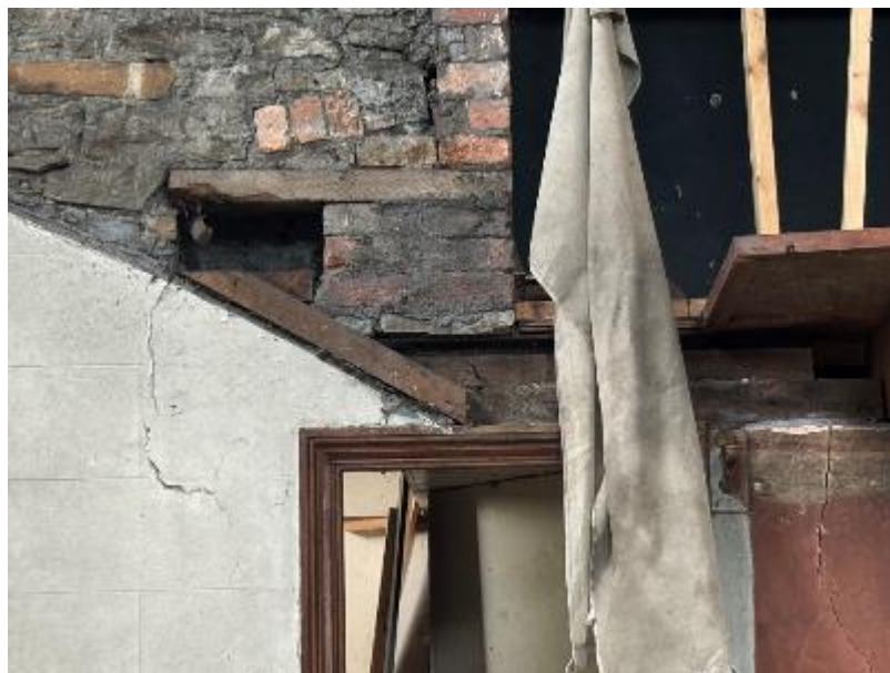
Photograph 12: Some localised cracking at the past beam end bearing locations
