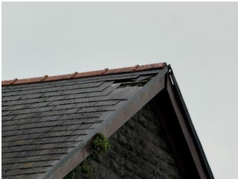
Photograph 21: Some missing slates to Main Chapel roof (West gable elevation)
