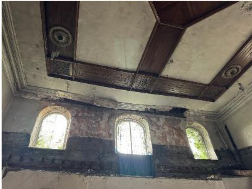
Photograph 20: Part damaged ceiling & cornice in the Main Chapel (likely due to water ingress)
