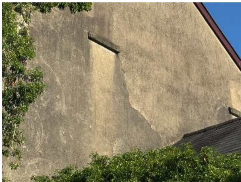
Photograph 27: Diagonal crack in the gable elevation wall
