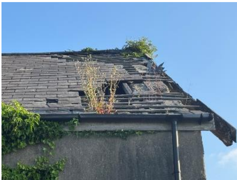
Photograph 6: Missing slates and damaged roof structure (Rear Extension)
