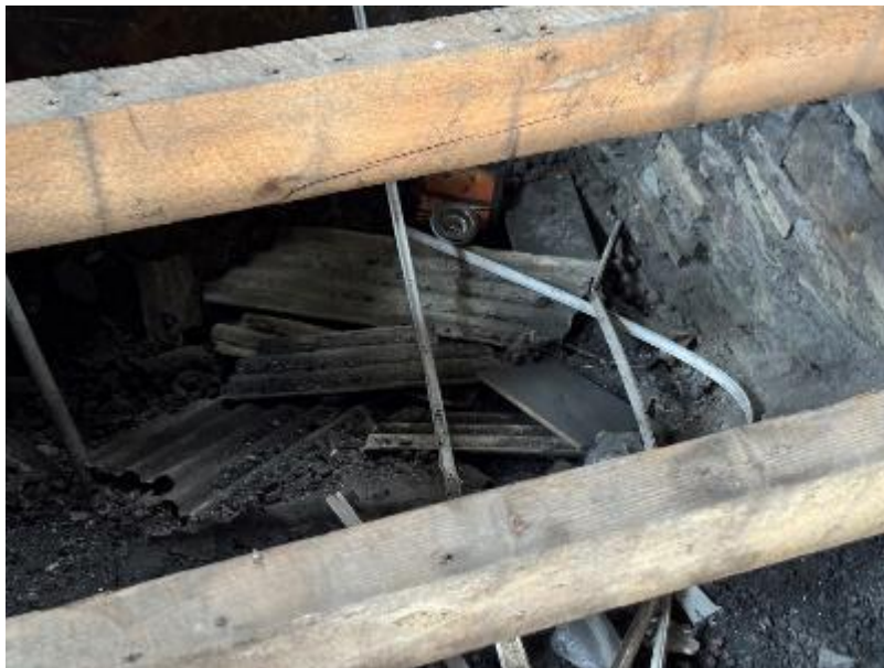
Photograph 15: Potential corrugated asbestos roof sheets
