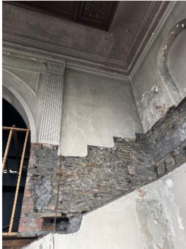
Photograph 11: Structurally distressed stone to the East gable elevation
