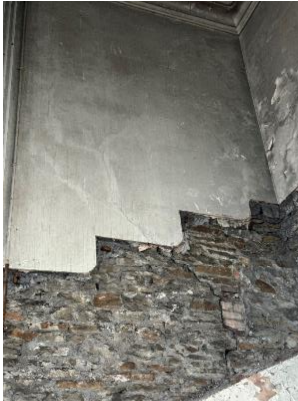
Photograph 13: Large vertical crack in the gable elevation wall
