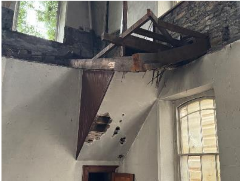
Photograph 16: Structurally unsound redundant timber stairs
