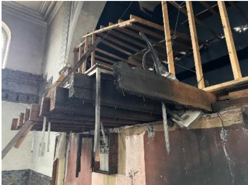
Photograph 17: Fire damaged structure
