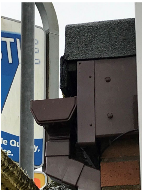
Photograph 4: Small gap under the apron at the south-eastern corner of B2.
