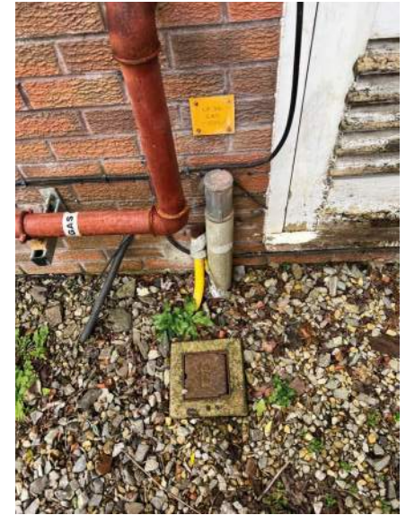
HP Gas Supply to Plant Room (East Elevation)
