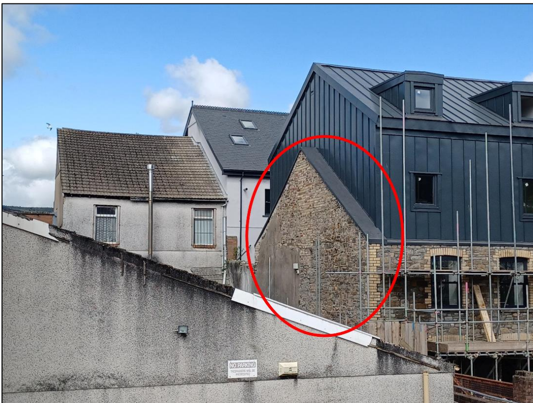
Photograph 5: Gable end of hotel where sand martins were observed entering gaps within the masonry.
