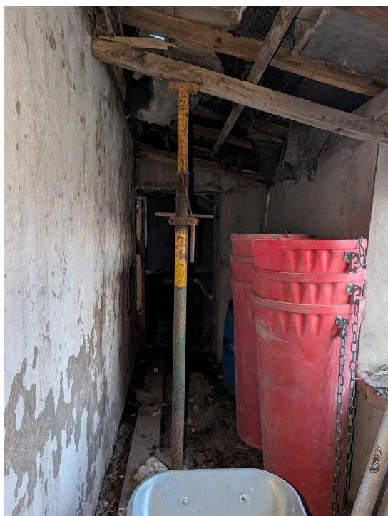
Plate 4 - Derelict internal area with peeling plastered walls, exposed ceiling timbers, an acrow prop and stored materials
