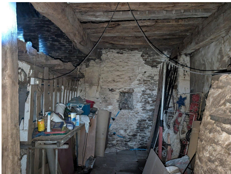
Plate 6 - Internal storage room with degraded plaster over stone walls, exposed ceiling beams, stored tools and materials and a blocked former opening.
