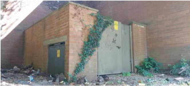
Existing Sub Station
