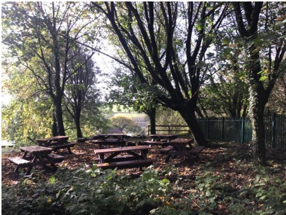
Image 4: Tree ID 2705. Heavily leaning tree over benches, remove for safety
