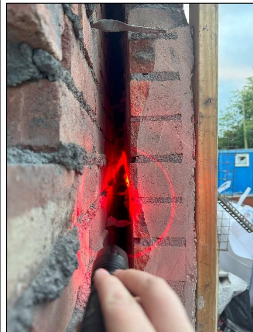
Plate 4 – The cobwebs within the cavity walls.
