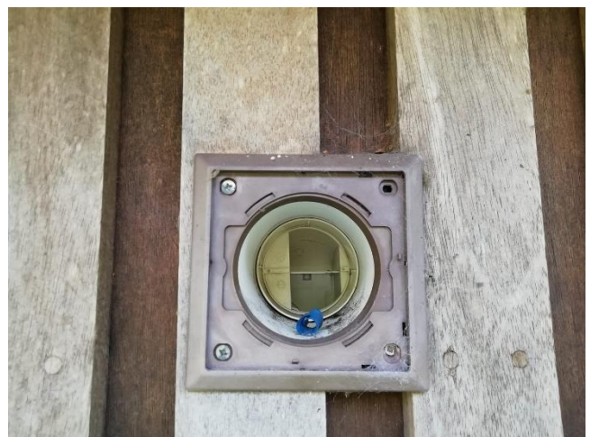
Figure 12 – Vent on pod does not open into a PRF
