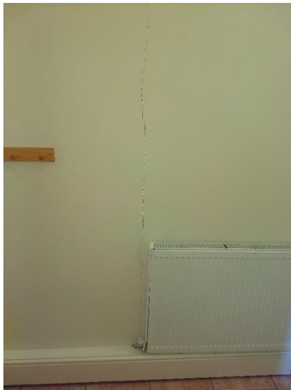
Photo 14 - Internal masonry wall, side facing the corridor. Gap below the skirtings and the floor ranging from 15-25mm max. Crack on the wall at the location of the blocked opening
