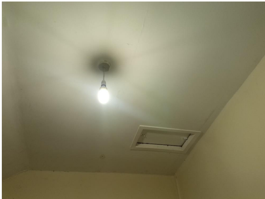
Photo 22 - Crack at the ceiling in the storeroom
