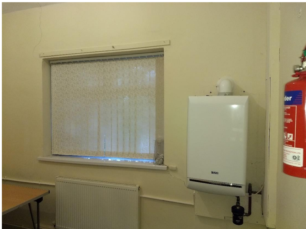
Photo 16 - Diagonal cracks at the top left and bottom right corner of the window in the storeroom (photos 17 & 18 show a closer view)
