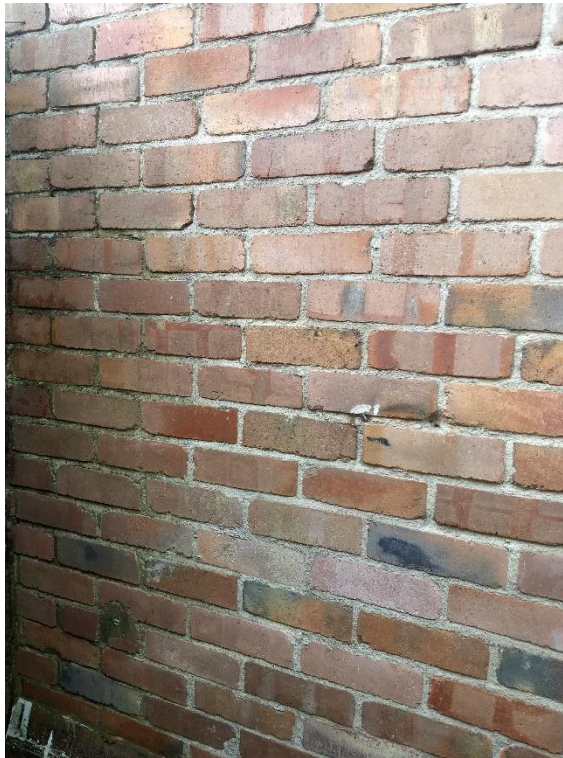
Photo 11 - External wall at left part of South East front elevation where partially filled joints are shown (Part 3)
