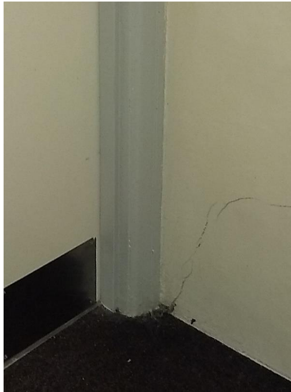
Photo 15 - Internal masonry wall, side facing the storeroom, with crack at the bottom corner
