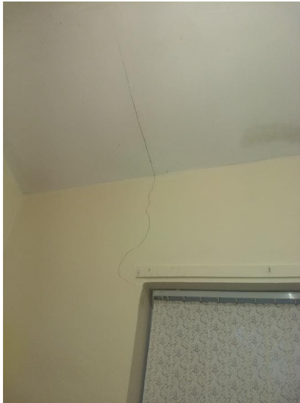
Photo 17 - Stress relief diagonal crack at the top left of the window in the storeroom
