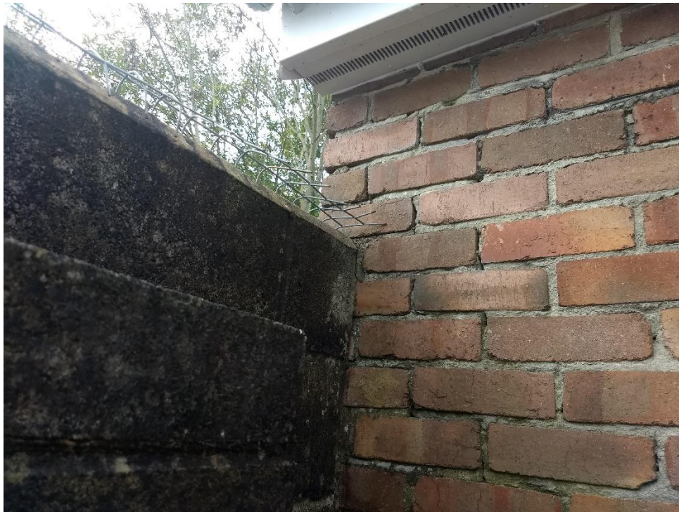
Photo 10 - External wall at top left part of South East front elevation where partially filled joints are shown (Part 3)
