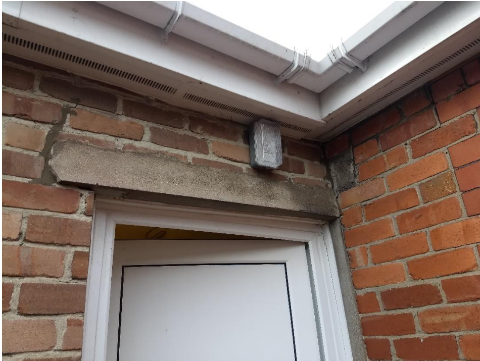
Photo 13 - Stress relief crack at the corner of the concrete lintel above the front entrance door
