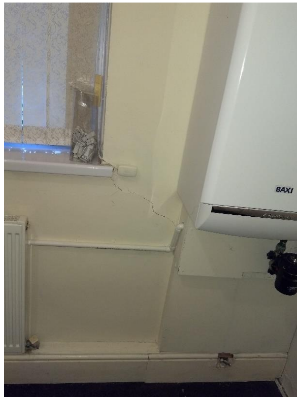
Photo 18 - Stress relief diagonal crack at the bottom right corner of the window in the storeroom
