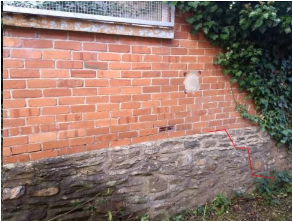
Photo 9 - Later built Part 2 North West elevation- cracks marked with red line indicating settlement, air brick showing.
