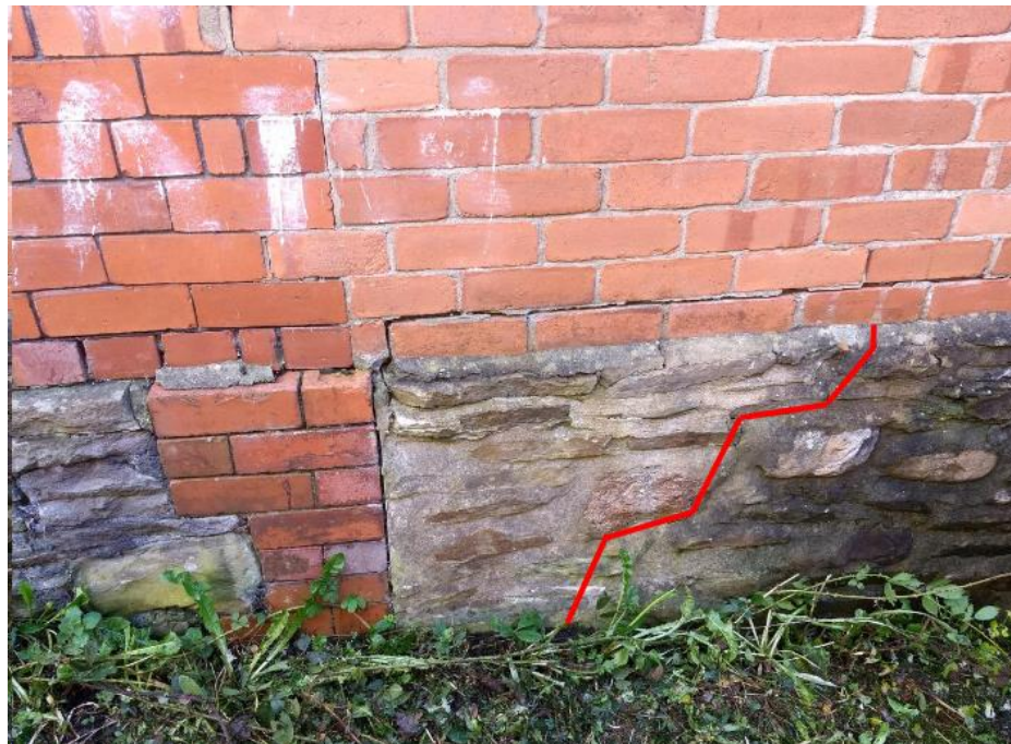
Photo 8 - Older Part 1 (left hand side) and later built Part 2 (right hand side) North West elevation- cracks marked with red line indicating settlement
