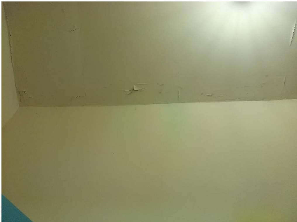
Photo 20 - Crack at the ceiling in male wet room
