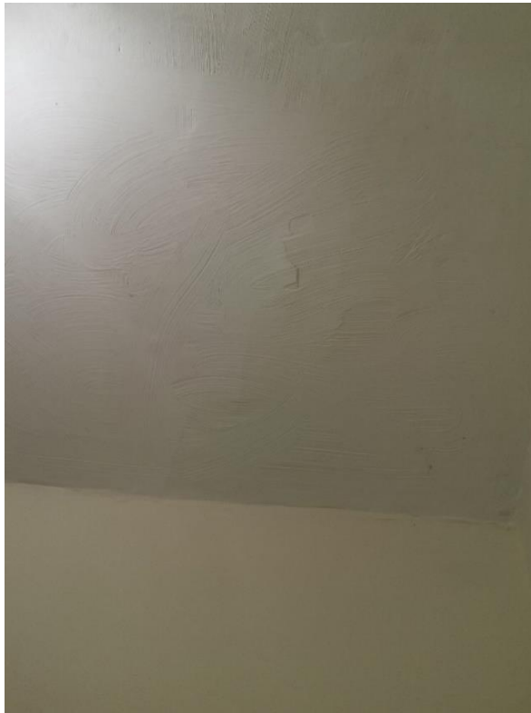
Photo 21 - Crack at the ceiling in female wet room
