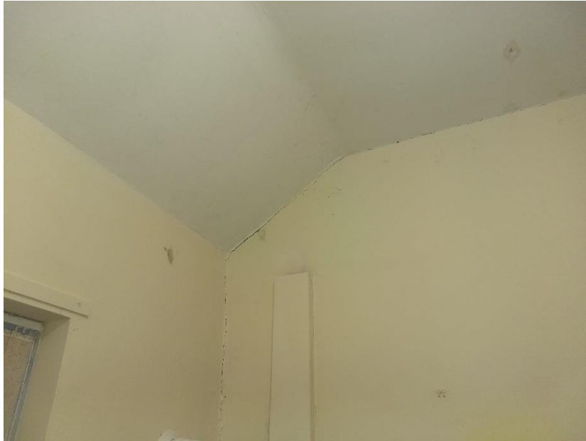
Photo 23 - Crack at the joint between the ceiling in the storeroom and the masonry internal and external walls
