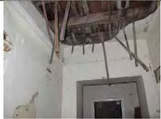
Damage to ceiling, interior of building
