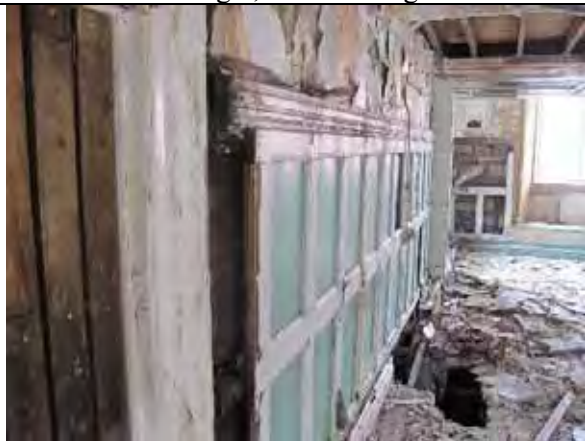
Water damage in building 1 interior
