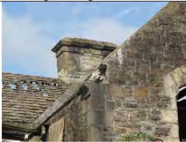
Damage to exterior stone work on western elevation
