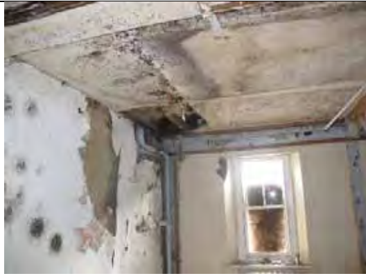
Interior of building 1, water damage
