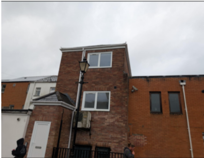
Plate 2- small gap beneath fascias
