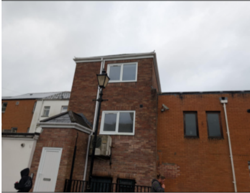
Plate 2- small gap beneath fascias
