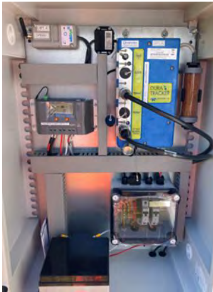
Figure 4: ISCO DuraTracker area-velocity flowmeter and Wildeye 4G Telemetry Datalogger assembly
